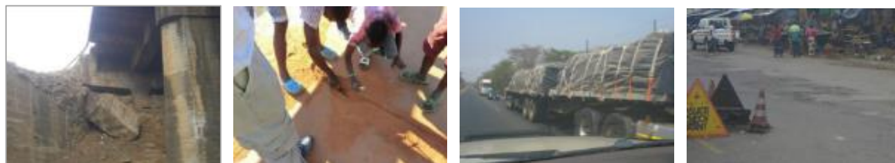
橋梁土台落下
