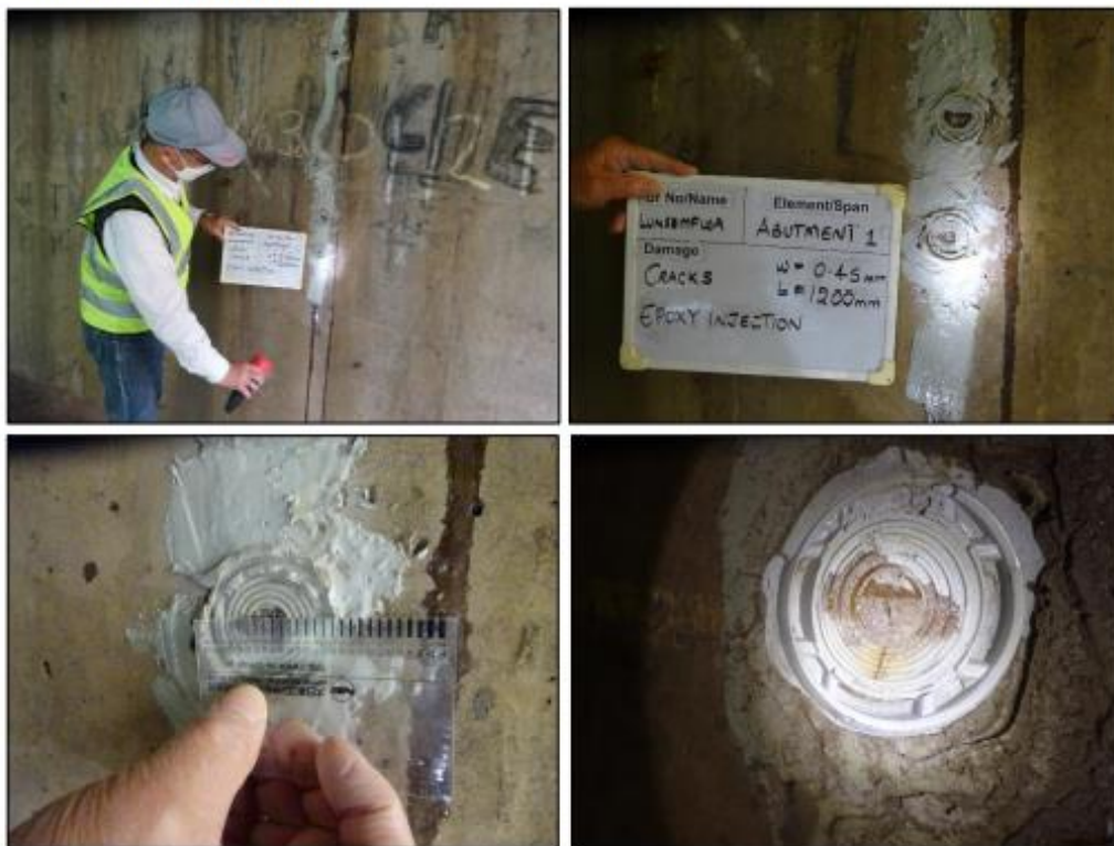
Photo 2: shows the condition of the Injection repair
