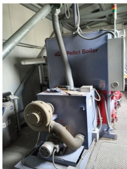
Pellet boiler introduced by this project
