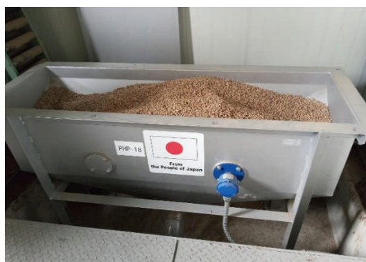
Photo 5: Pellet fuel before use (Primary school in Chiperceni)
