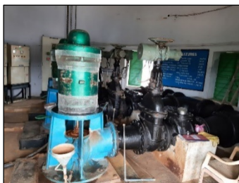
Pumping Facility (Tiruchirappalli)
