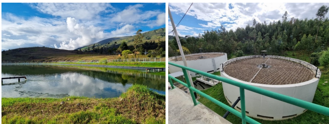
STPs constructed and in operation under the Project
