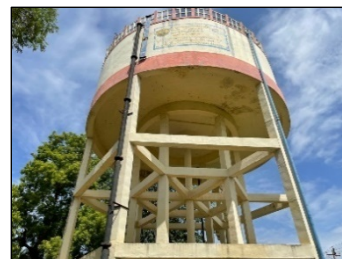
Water Storage Facility (Devakottai)
