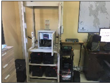
Photo 1: Strong Motion Seismometer (Region VIII Leyte, Palo earthquake monitoring station)
