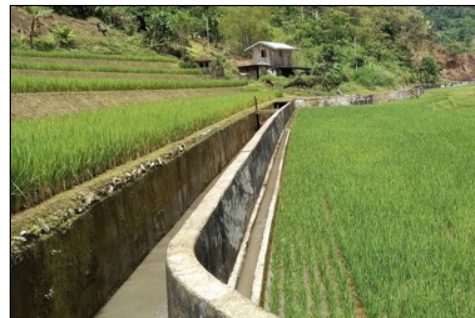
Headrace. The narrow canal on the valley side is the rehabilitated irrigation channel.
