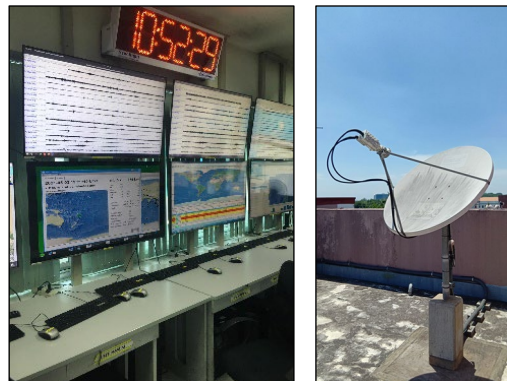
Equipment maintained by this project (PHIVOLCS headquarters monitors, IPSTAR satellite communication equipment)
