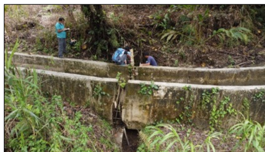
A damaged part of the headrace. A part that was repaired in the past was damaged again.
