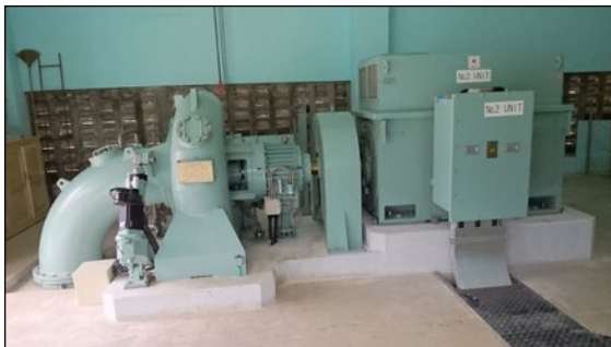
Water Turbine and Generator
