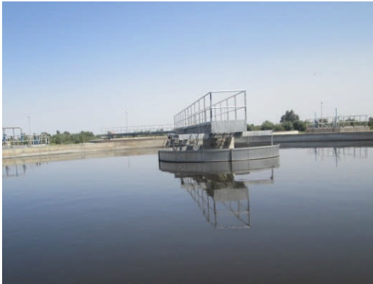
Sewage treatment facility developed by this project (El Kelaa des Sraghna City)
