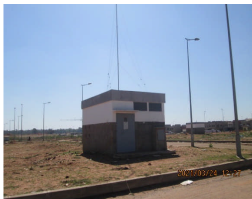
Developed substation equipment
