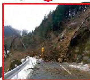
Road is disconnected by slope failure.
