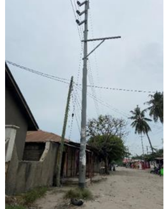
33kV Distribution line
