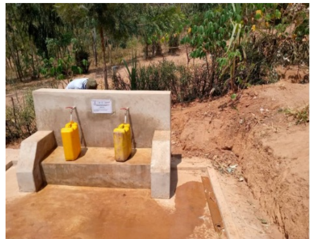
Public water tap installed by the district by extending the distribution pipeline from the project facility (Remera Sector, Gatsibo District)
