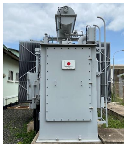
33/11kV Transformer (Msasani substation)
