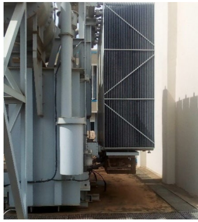
Grounding part of transformer
