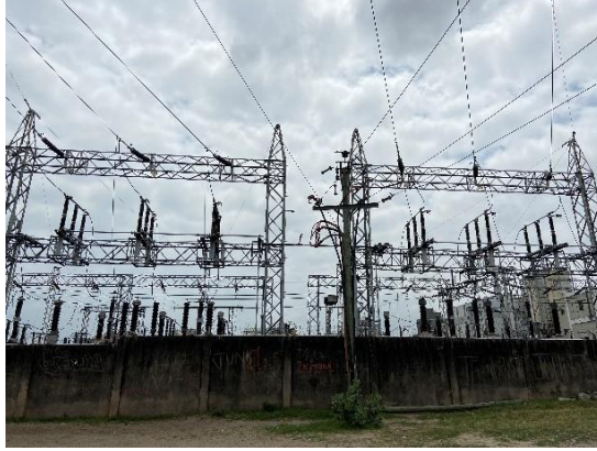
132kV Transmission line gantry (Ilala substation)
