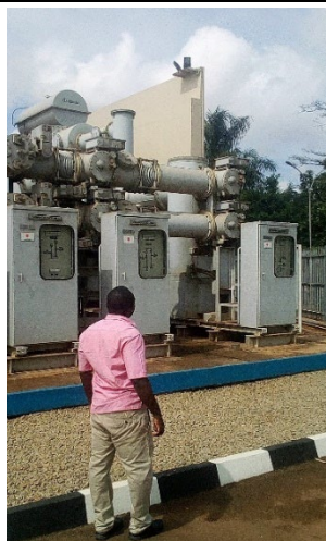
Outdoor 132 kV gas insulated switchgears
