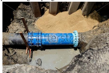
Repairing metallic pipe by flanged connector in one side and dismantling joint in another
