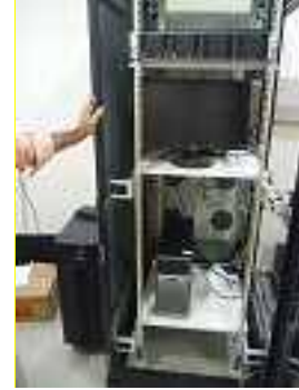
P-6: Server (Data transmission equipment to existing financial system)
