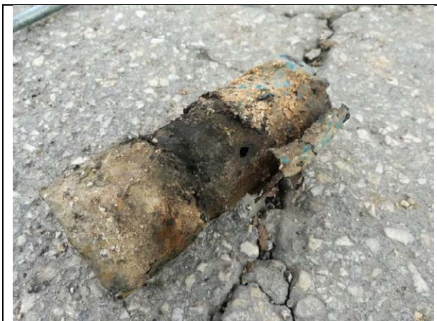
Photo 3.5 Cause of Leak (pin hole in the pipe)
