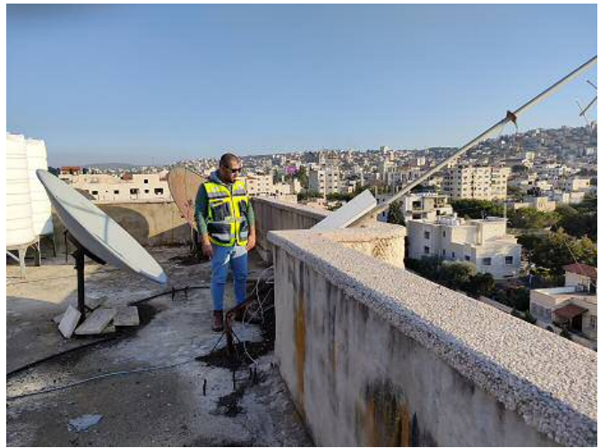
Photo 6.2 GW installed at the roof top of a building
