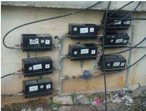
Photo 6.4 PPWMs installed at the apartment
