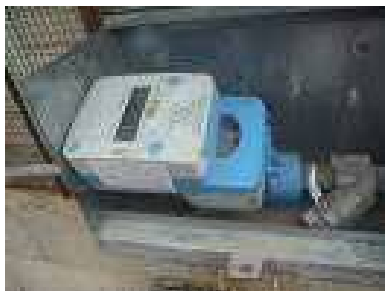
P-1: PPWM installed at household
