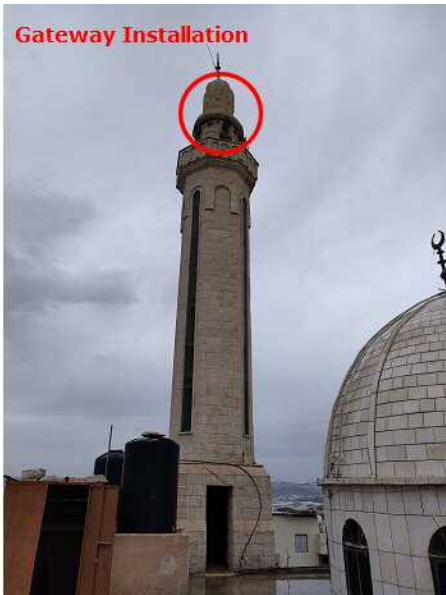
Photo 6.1 GW installed at a Mosque tower
