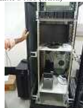
P-6: Server (Data transmission)
