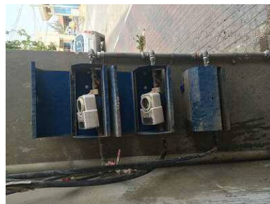
P-1: PPWM installed at household
