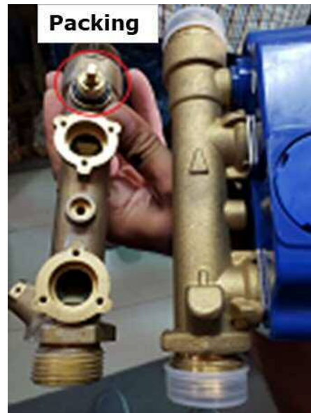
Photo 10.2: The part through which water leaked into PPWM
