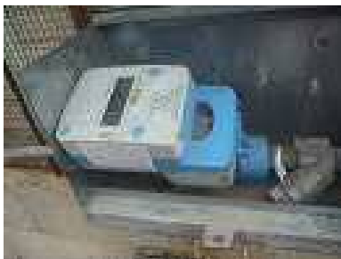
P-1: PPWM installed at household
