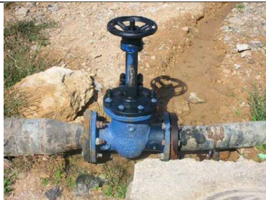
Leakage from improperly welded pipe
