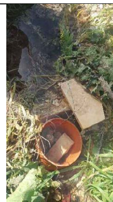
Leakage from a valve in Sabah Al Khir area
