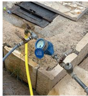
0- meter reading visit- broken meter and new meter after replacement
