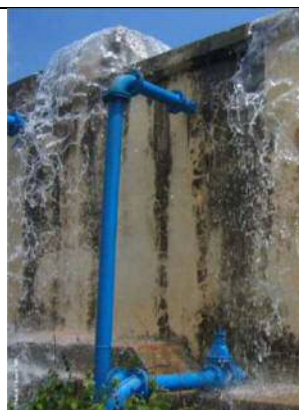
Overflow from water utility tank
