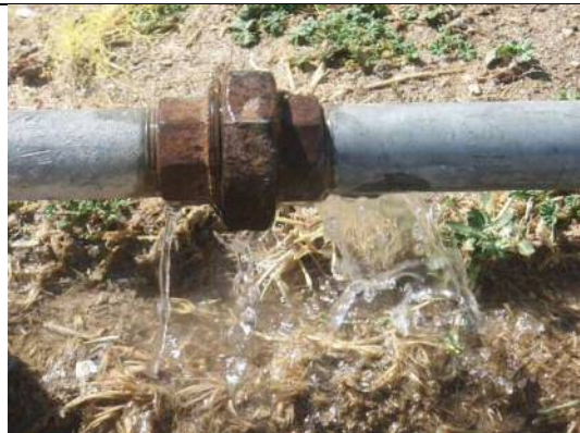
Leakage from improperly connected pipe
