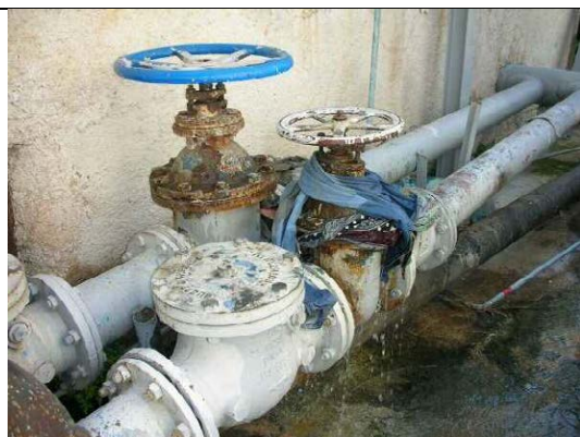
Leakage due to inadequate maintenance of valves
