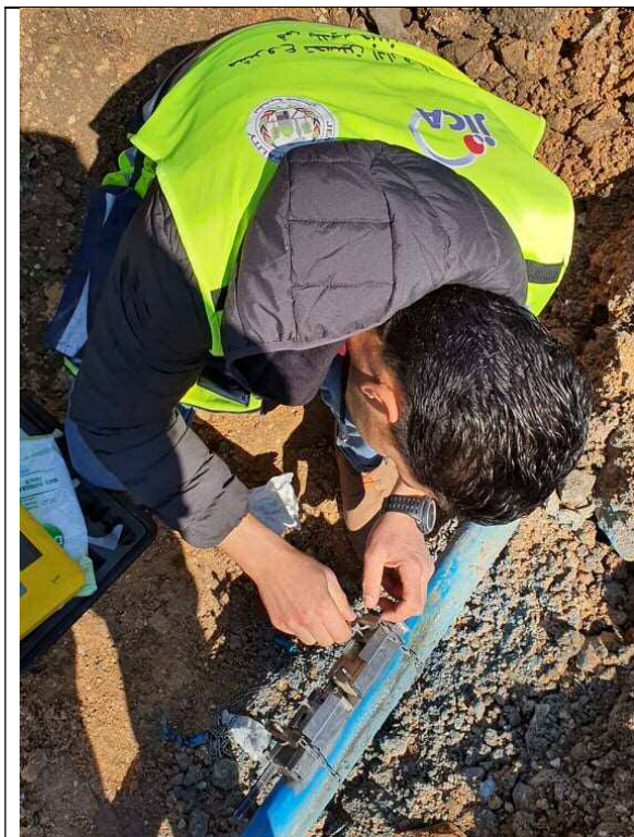
Attaching the sensors
