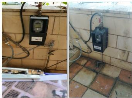
Sample Illegal Connection at PPWM; before and after
