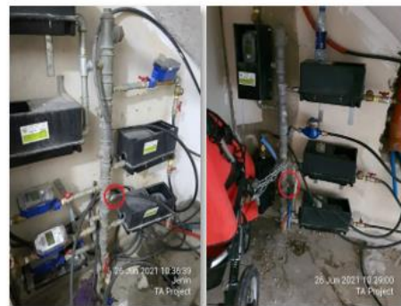
Some other Illegal Connections
