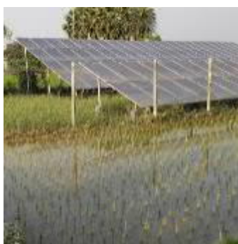
Solar Panel for Irrigation
