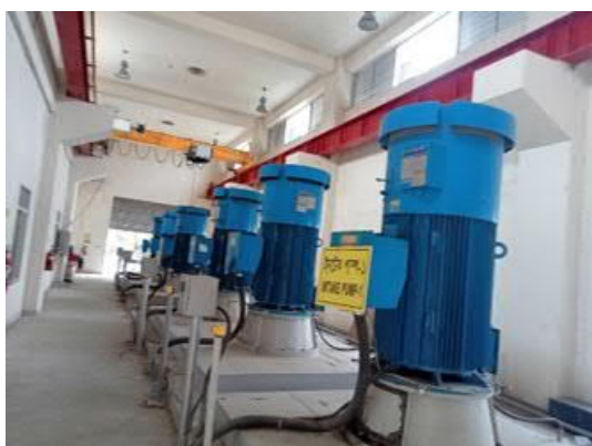
Photo 2. Pump station at Karnaphuli water intake facility (photographed by a local assistant in June 2021)
