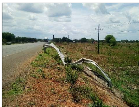
Damaged guardrail (4.6 km from Elegu)
