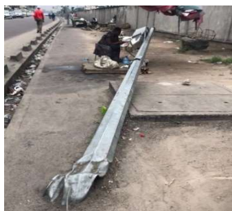
A collapsed streetlight left unattended
