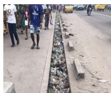
Garbage filling the side ditch
