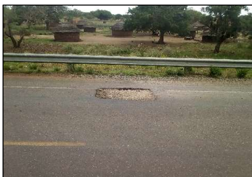
Pothole (10 km from Elegu)
