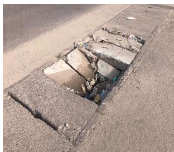
Damaged concrete side ditch covers
