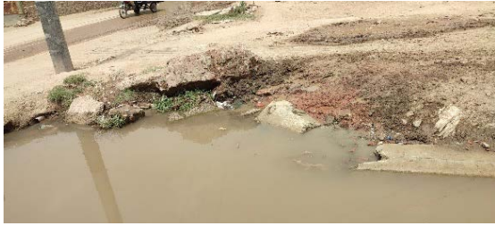
Figure 9. Damaged Side Protection at Tulwala Distributary
