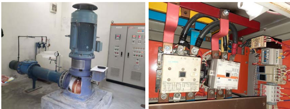
Tubewell constructed by the Project (right: inside of control panel, left: pump)
