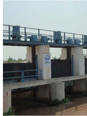
Figure 10. Damaged Cross-regulator Cable at Burala Branch
