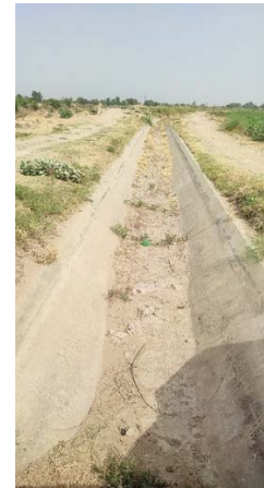
Figure 8. Insufficient Water Supply at Minor
