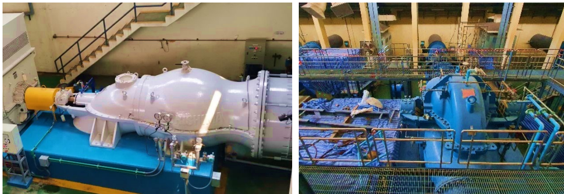
Raw water pump (left) and transmission pump (right) at Bangkhen WTP
