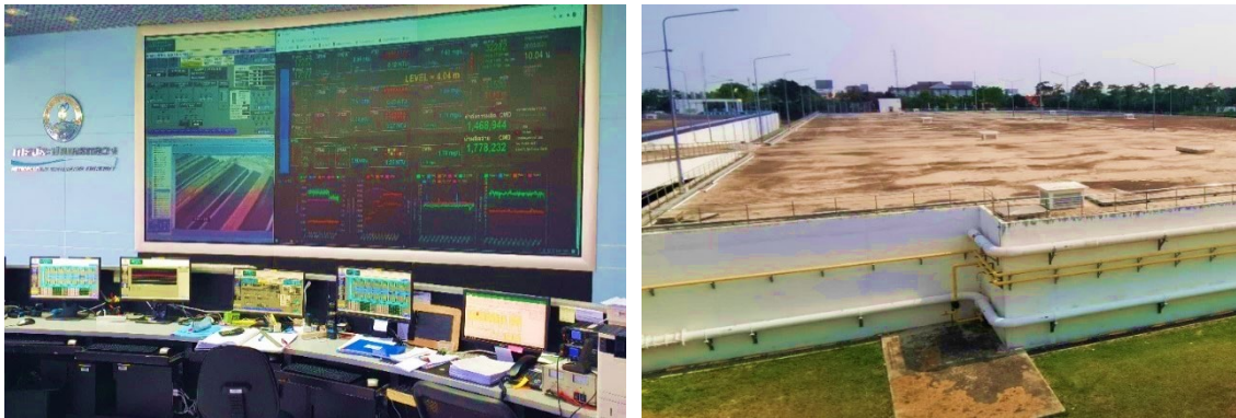
SCADA system 5 (left) and reservoir (right) at Mahasawat WTP
