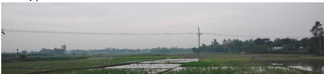
Photo Newly Constructed Medium- and Low-Voltage Lines (33 kV Line) (Rangpur Division, Dinajpur PBS-2)
