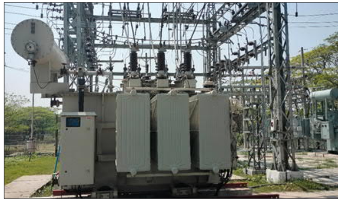
33/11kV Substation (Barisal Division, Patuakhali PBS, Golachipa Substation)
