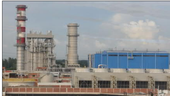
New Haripur Power Plant
