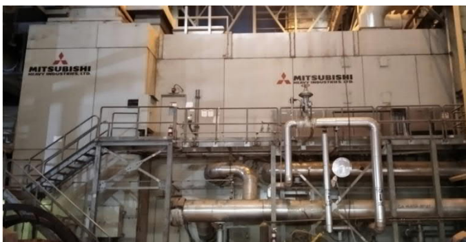
Photo: Gas Turbine
