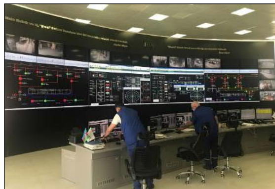
Right photo: Control room
