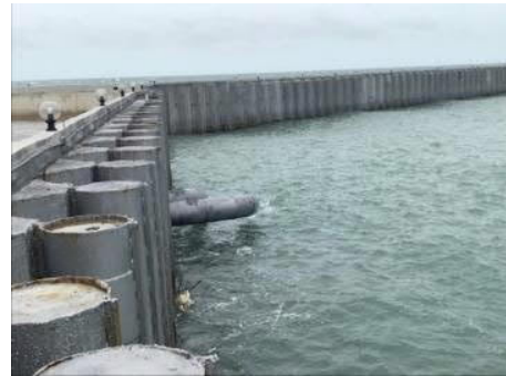
Photo: Pond-type water intake
