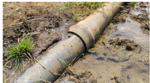
Water leakage between pipes
