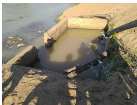
During floods, the water intake point is filled with sediment, making it difficult to take water. In addition, the pump is currently dysfunctional.
