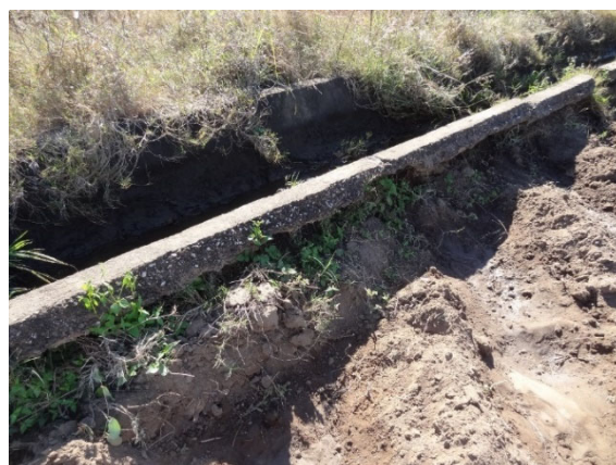
Figure 5.3.16 Spilling Out of Canal Back Side Soil
