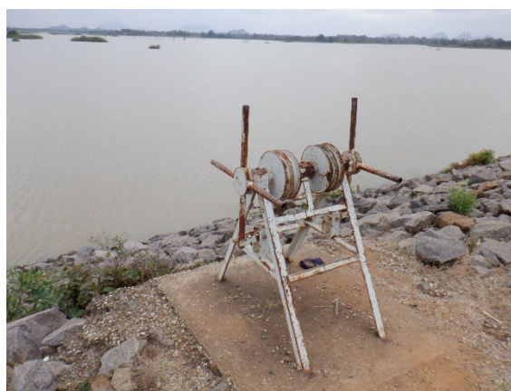
Figure 5.3.30 Winch for Intake Gate Operation
