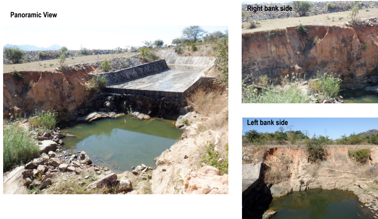
Figure 5.3.43 Collapse of Side Walls on Both Bank Sides at the End of the Spillway Channel
