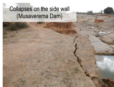
Figure 5.5.3 Deteriorations/Damages on the Connection Canal to be Treated by Zimbabwean Side
