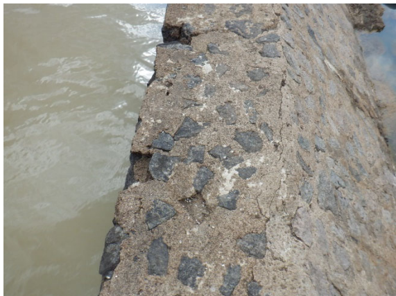
Figure 5.3.26 Surface Peeling and Lack of Stones
