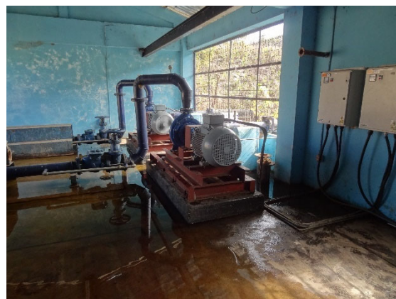
Figure 5.5.20 Status of the Pump Facility (Chinyamatumwa Dam)
