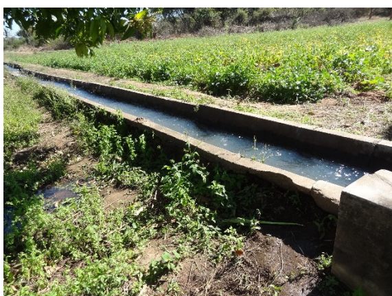
Figure 5.3.57 Spilling Out of Back Side Soil
