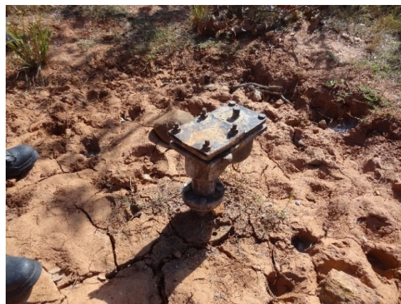
Figure 5.3.47 Mark of Water Leakage from Air Valve
