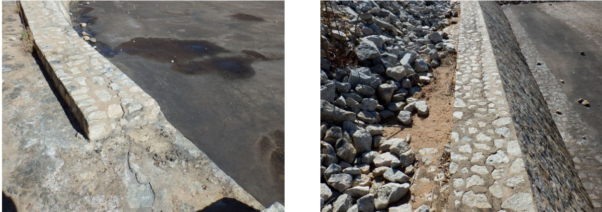
Figure 5.3.75 Cracks at the Top of Retaining Walls
