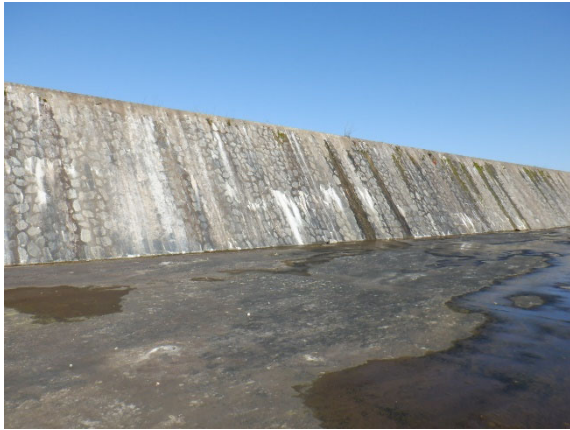
Figure 5.3.73 Leakage from Downstream Slope
