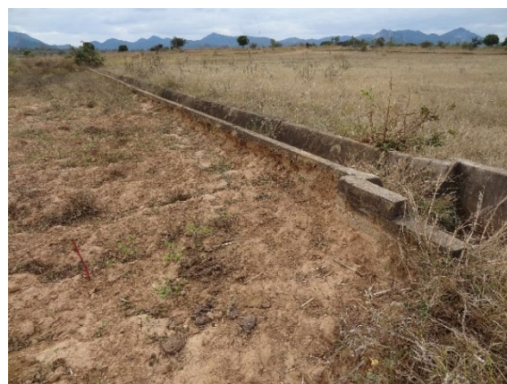
Figure 5.3.48 Silling Out of Back Side Soil
