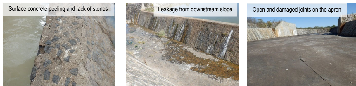
Figure 5.5.1 Deteriorations/Damages on the Spillway to be Treated by Zimbabwean Side
