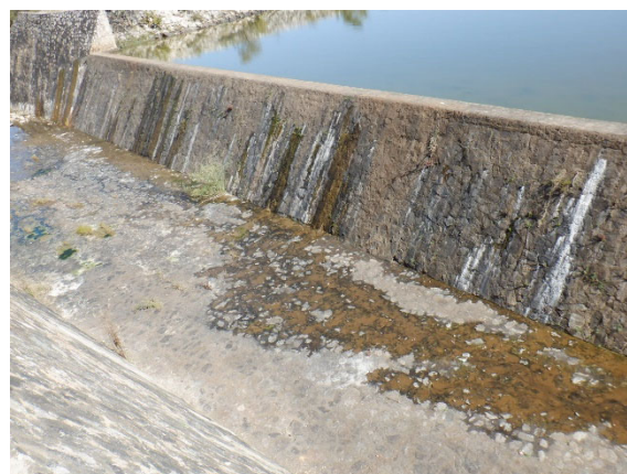
Figure 5.3.42 Leakage from Downstream Slope
