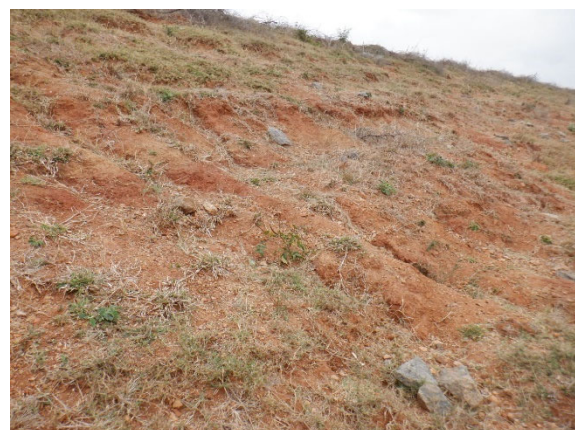
Figure 5.3.23 Gully Erosion (Downstream Slope)
