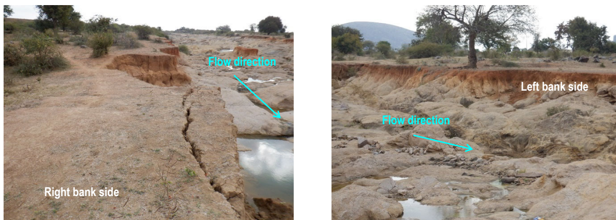
Figure 5.3.28 Collapse of Side Walls on Both Bank Sides
