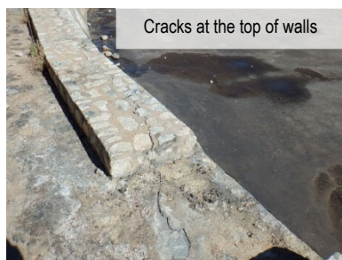
Figure 5.5.2 Deteriorations/Damages on the Spillway Canal to be Treated by Zimbabwean Side
