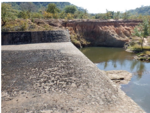
Figure 5.3.66 Collapse of Left Bank Side Wall at the End of the Spillway Channel
