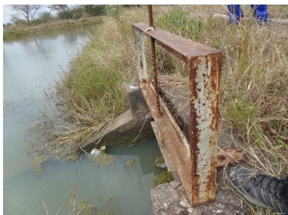
Figure 5.3.31 Broken of the Discharge Gate
