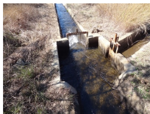
Figure 5.3.79 Broken Sluice Gate
