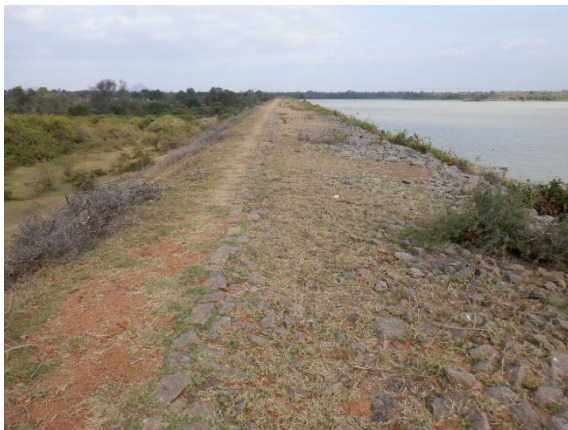
Figure 5.3.22 Disturbance of Riprap, Dam Body Exposure, and Erosion (Crest and Upstream Slope)
