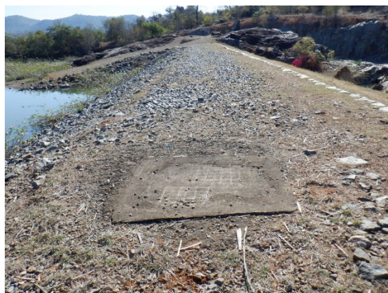
Figure 5.3.14 Disappearance of the Intake Gate Operation Facilities
