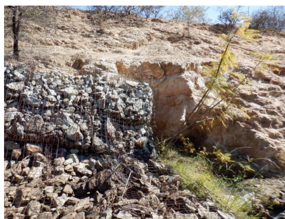
Figure 5.3.77 Collapse of Left Side Bank
