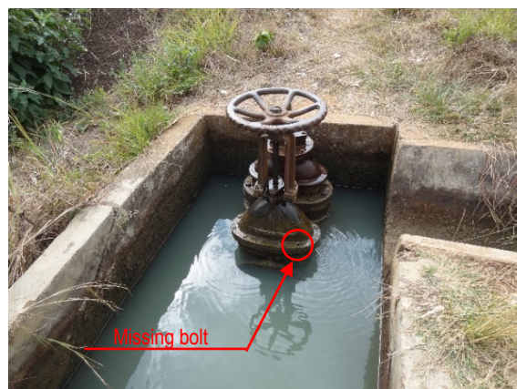
Figure 5.3.32 Missing Parts of Sluice Valve
