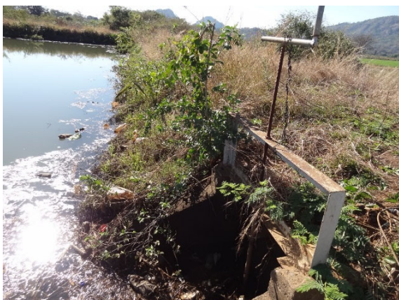
Figure 5.3.15 Broken of the Discharge Gate
