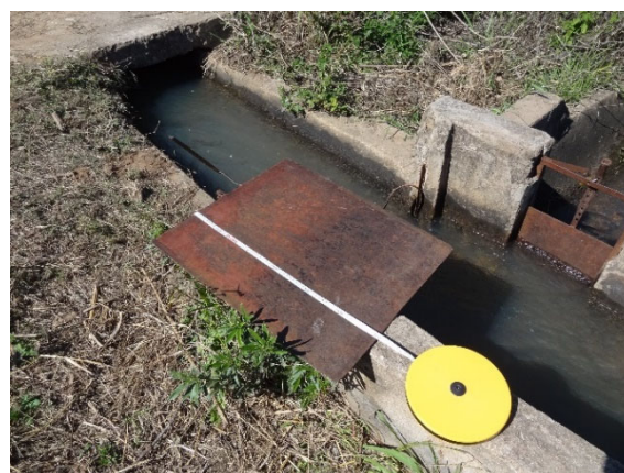
Figure 5.3.58 Broken of Sluice Gate
