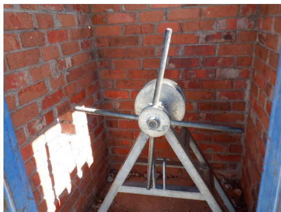
Figure 5.3.78 Winch on the Crest
