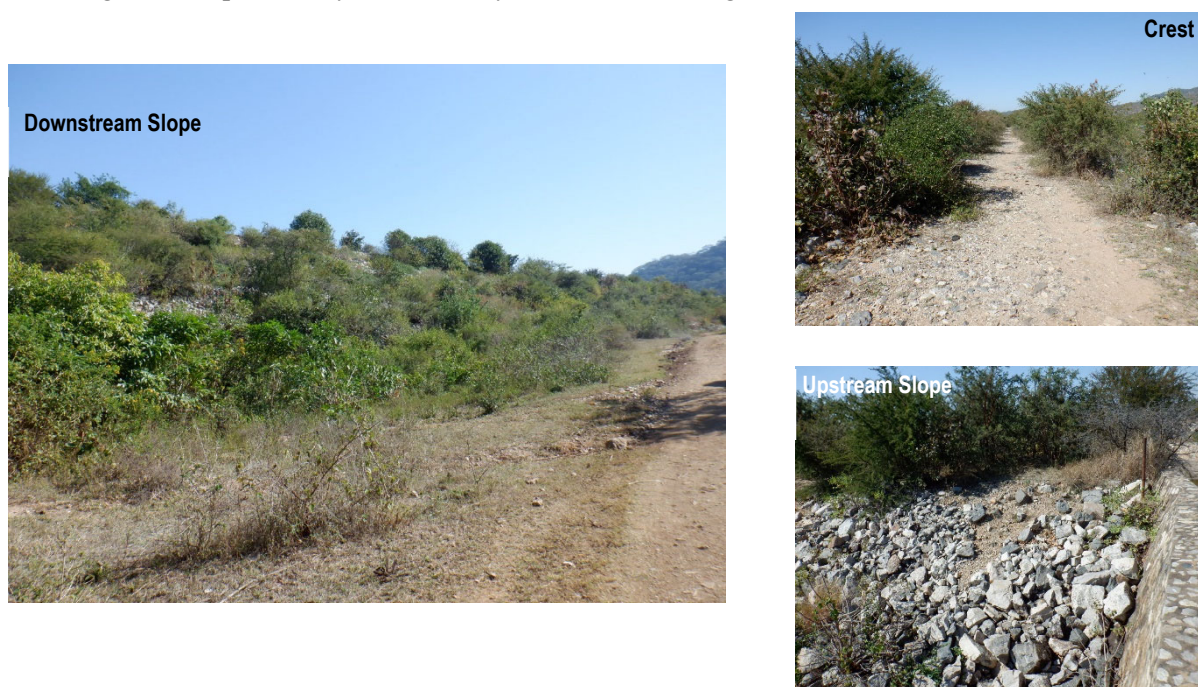
Figure 5.3.54 Partial Disturbance of Riprap, Dam Body Exposure, and Many Trees
