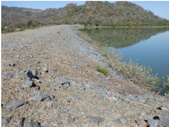
Figure 5.3.5 Disturbance of Riprap, Dam Body Exposure, and Erosion (Crest and Upstream Slope)
