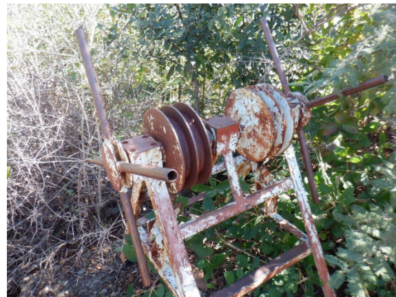
Figure 5.3.56 Winch for Intake Gate Operation
