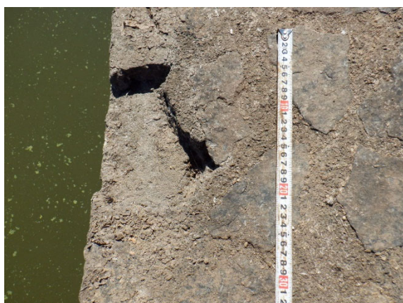
Figure 5.3.41 Slight Damage on the Crest
