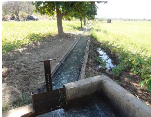
The back soil is flowing out. OF(10):On farm canal(4)
