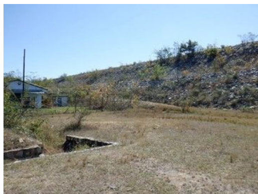
D(2) Embankment Dam body exposure, gully erosion under riprap, and trees.
