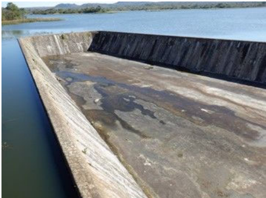
S(1) Spillway entire: No significant damage is observed. The abutment is flat.
