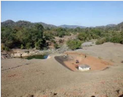
C(7) Connecting Canal: The erosion on the right bank side has reached the slope of the valve house.
