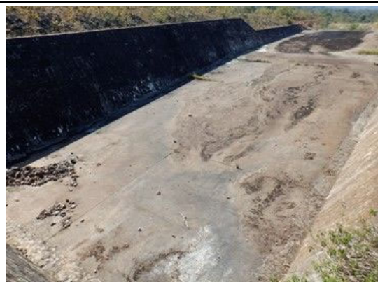
S(5) Spillway Apron: No scour is observed, and small rocks, plants, and open joints can be observed.
