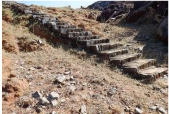
D(4) Embankment Downstream: Erosion is also observed on both sides of the stairway on the left bank.
