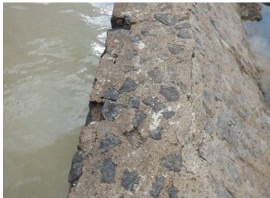
S(3) Spillway weir: Surface peeling and lack of stones on the top
