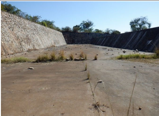
S(5) Spillway Apron: A few rocks and cracks are observed on the bottom. There is no scouring at the bed. Low plants in joints.
