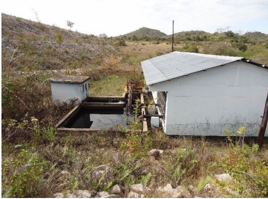
PS(1): Full view of pump station
