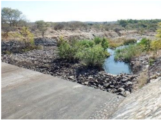
C(1) Connecting Canal: The right side of the gabions (t50cm) has been washed away.
