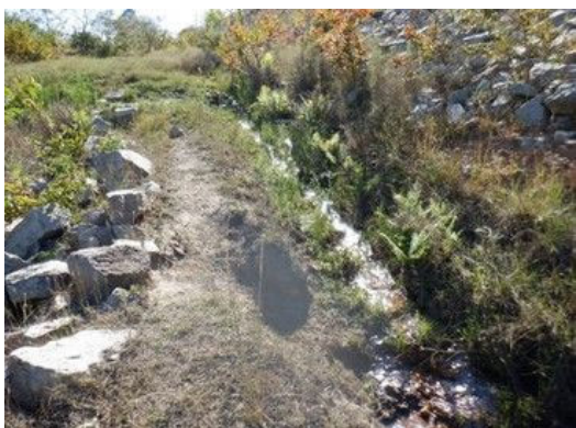
D(5) Embankment Downstream(right): Seepage and slight flow at the downstream slope edge.
