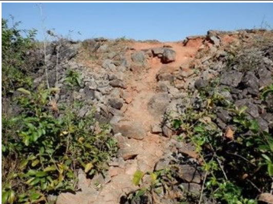
D(5) Embankment Downstream: Riprap is disturbance and dam body is exposed near the crest, edge, and paths. Many trees in the left side.
