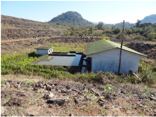
PS(1): Full view of pump station
