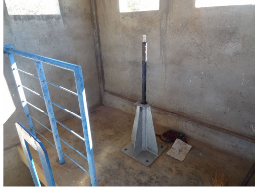
I(2) Intake Outlet: The handle has been vanished away.
