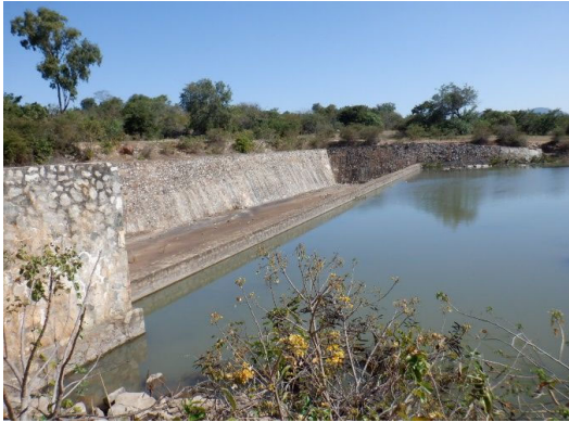
S(1) Spillway over view: No significant damage.
