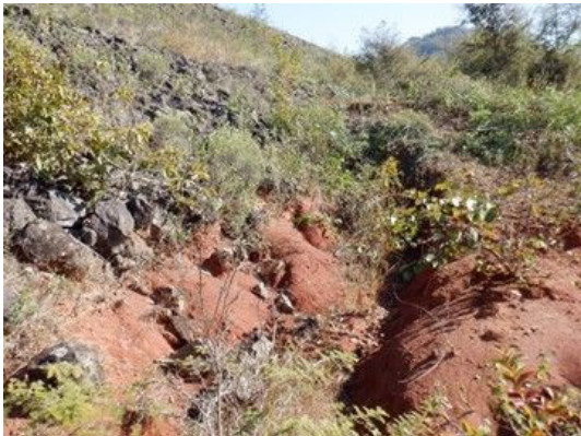
D(3) Embankment Downstream(left): At the slope edge, there are flow route and those eroded the edge. (No flow or wetness.)
