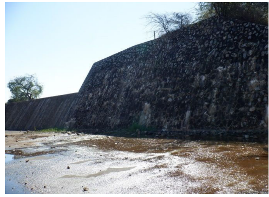
S(4) Spillway Retaining wall (left): Efflorescence from cracks (not draining from drainage holes).
