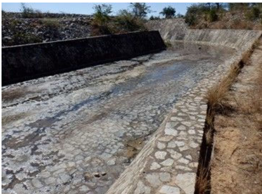
S(7) Spillway canal: Small rocks, a slight plants, and some water are observed.
