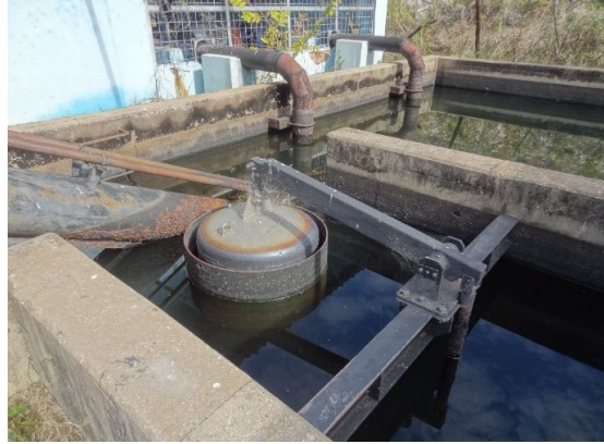
Rusted float valve
