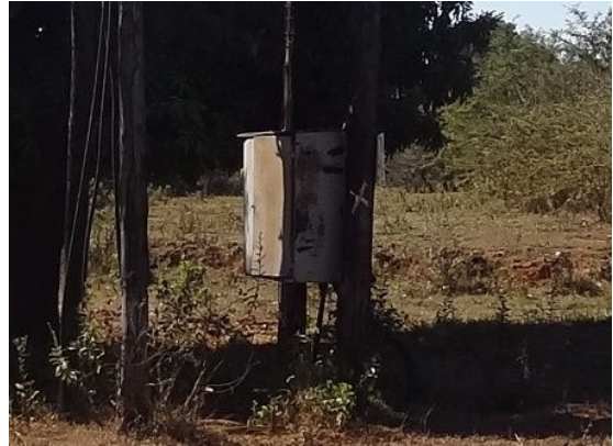
PS(8):Power receiving board
