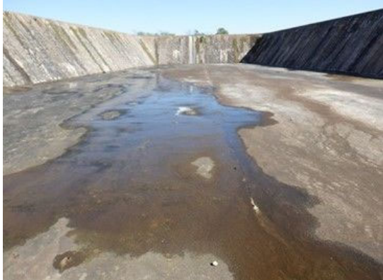
S(5) Spillway apron : No cracks, plants, or washes are observed.
