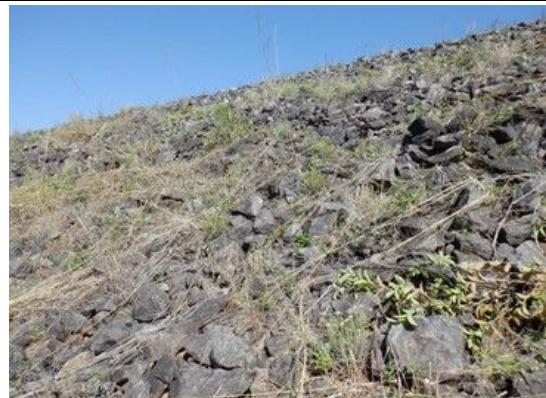
D(6) Embankment Downstream: Gully erosion under riprap makes downstream ditch which is filled with rocks. Lower those area, dam body is exposed but there is no seepage.
