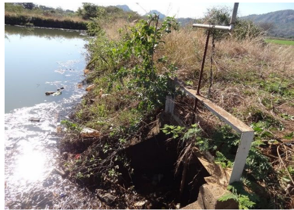
The upstream gate has broken.
