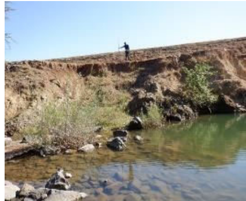
C(4) Connecting Canal: The large erosion on the right bank side (embankment side) extends beside of the valve house.
