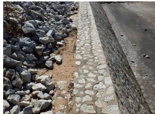
S(4) Spillway retaining wall (left): There is a crack less than 1cm width on the top of the retaining wall. (L10m).
