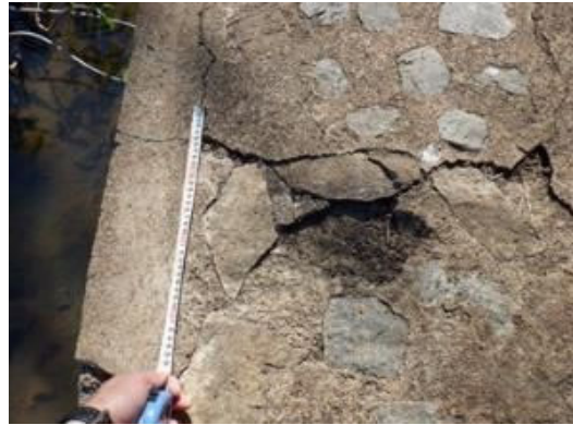
S(2) Spillway Weir: Surface concrete peeling at the top of the weir.(L7.5m/t5cm)
