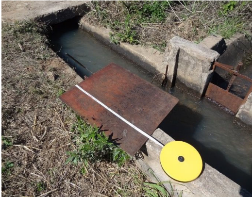
Gate has been broken. (H600xW520) OF(7):Diversion(1)
