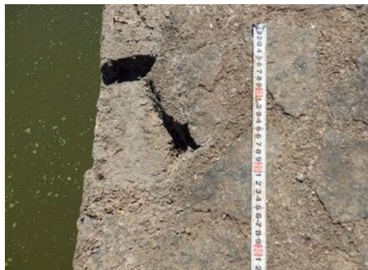
S(2) Spillway weir: Slight damage on the crest.
