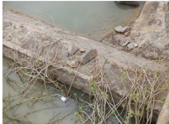
S(2) Spillway weir: Surface peeling and lack of stones on the top
