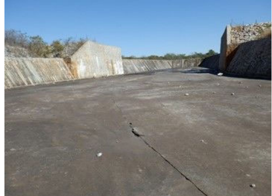
S(6) Spillway apron : Opening of joints (up to 3cm, detached joint material), damage to joints (60cm, 40cm), and small stoners are observed.
