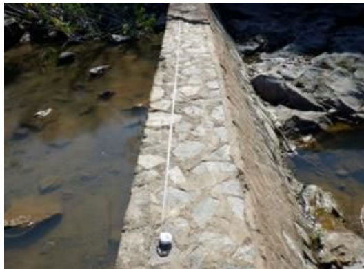
S(3) Spillway Weir: Surface concrete peeling at the top of the weir.(L7.5m/t5cm)
