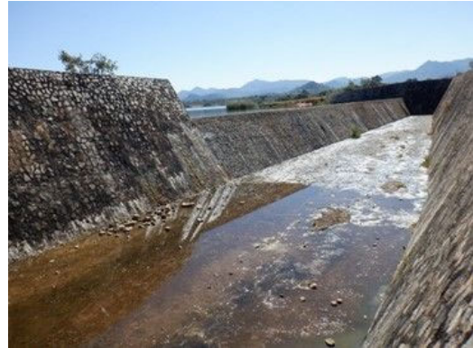
S(4) Spillway apron: Small rocks, a slight plants, and some water are observed.
