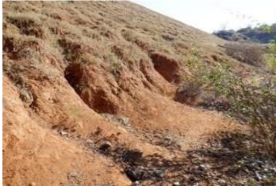
D(7) Foot of slope: There are collapses due to erosion (the height of the collapses are 1.7m and 1.2m at the largest).
