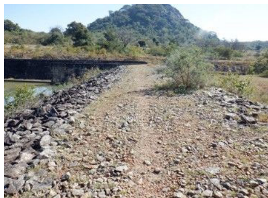
D(10) Crest of Embankment: Tree in the left side.
