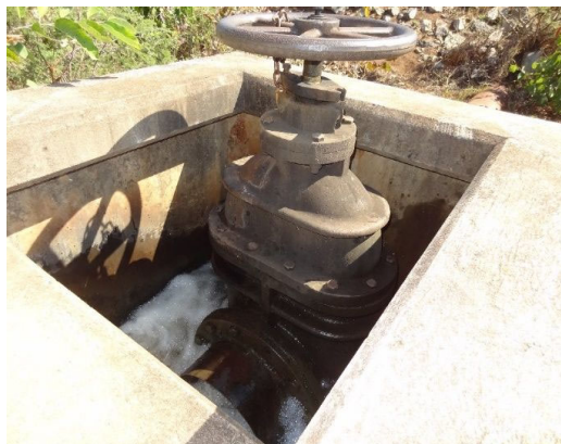
The valve is movable and in good condition. OF(3):Night storage(Outlet valve)
