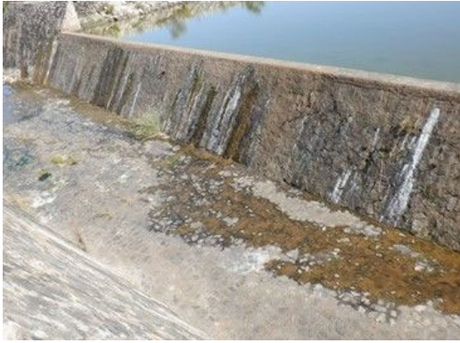
S(3) Spillway weir: Leakage on the downstream side
