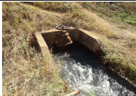
The downstream valve is movable and in good condition.
