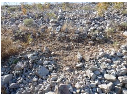
D(3) Embankment Downstream: Below the first step, there are several sinks (collapsed embankment material is filled with rock material. The largest one is about B2.0m.). In the lower part of it, the soil is exposed in some places.
