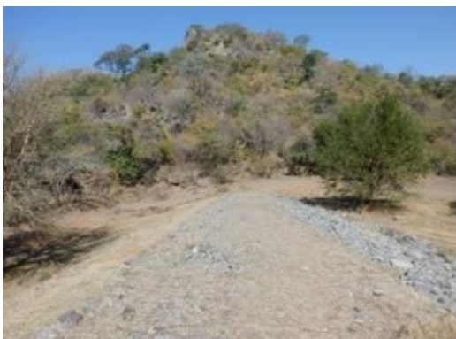
D(11) Right side abutment: There is no disturbance in the abutment. The land is high mountain. There is farmland on the downstream side.
