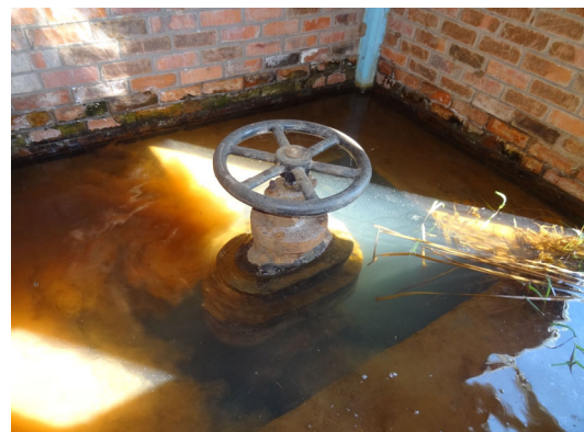
I(2) Intake Outlet: The valve has movable and submerged.
