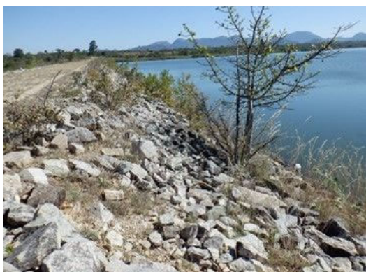
D(1) Embankment Upstream: Dam body exposure, gully erosion under riprap, and trees.
