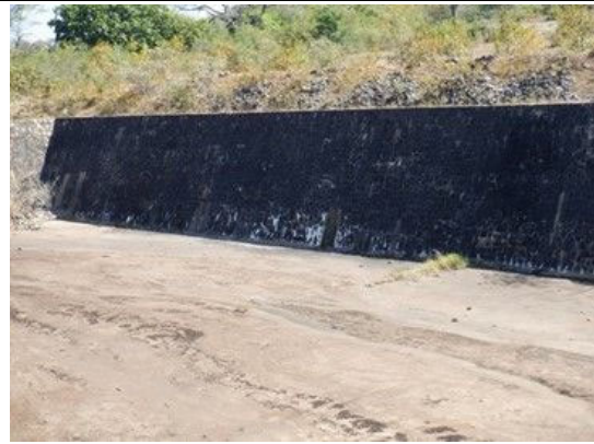
S(8) Spillway Retaining wall(left): Efflorescence is observed. On the left bank side, leakage of seepage water from the ground (water can be seen, but there is no flow).
