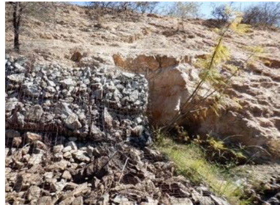
C(4) Connecting Canal: Downstream of the gabions, there is a collapse on the left side (L1.8m, B1.2m, H3.0m).
