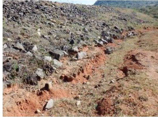
D(2) Embankment Downstream(right): At the slope edge, there are flow route and those eroded the edge. (No flow or wetness.)
