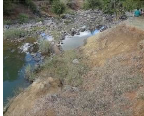
C(6) Connecting Canal: The canal bed has been eroded and the concrete siphon protection are exposed.
