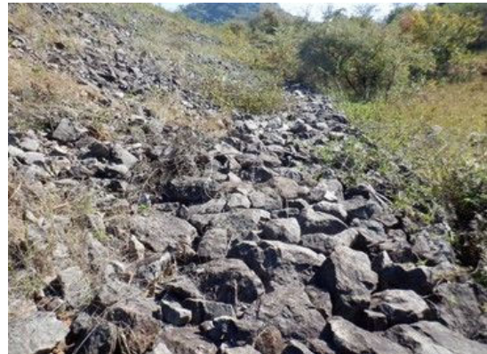
D(4) Embankment Downstream: Riprap is disturbance and dam body is exposed near the crest, edge, and paths. The stone is not stable and hard to walk on.
