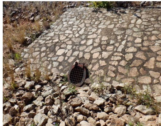
Good condition. OF(4):Night storage(Distribution hole)
