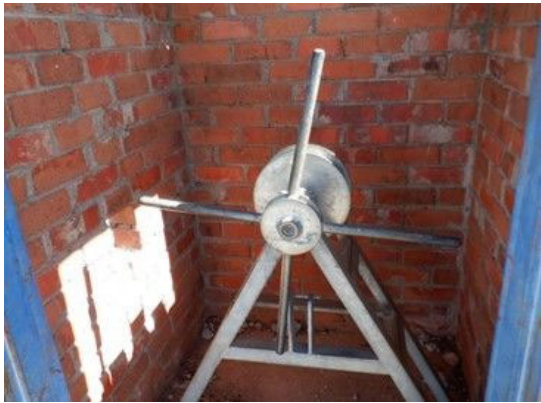
I(1) Intake Inlet: The building and winch are located at the crest, but the wires have disappeared. The handle can be turned.
