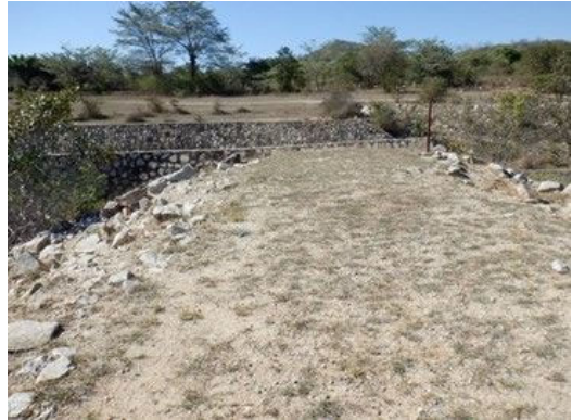
D(10) Left side abutment: No significant damages are observed at the boundary with the spillway. Elevation difference is small (hill-like terrain) . There is farmland in the upstream side.
