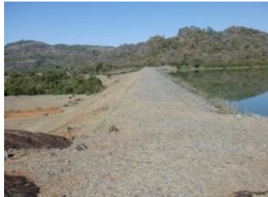
D(6) Crest of Embankment: Disturbance of riprap, dam body exposure and erosion.
