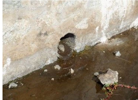
S(8) Spillway canal: The bottom of the drainage hole at the bottom of the retaining wall is wet.
