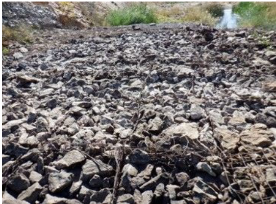
C(3) Connecting Canal: The cages are damaged. It is used as a walkway for crossing.
