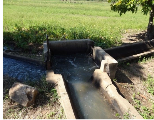
A small amount of water leaks, but there is no problem. OF(8)Diversion(2)
