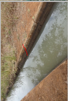
There are some cracks around the crest.
