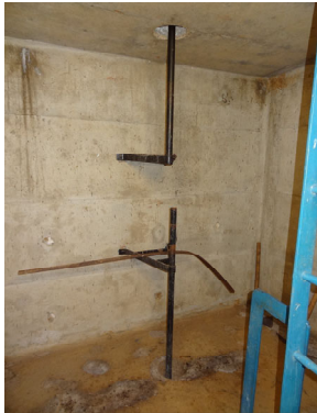
I(3) Intake Outlet: The middle of spindle had been broken.
