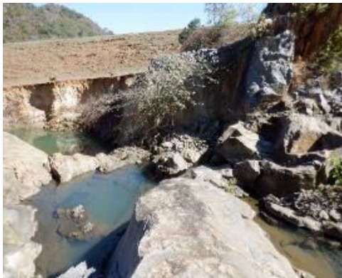
C(1) Connecting Canal: The large erosion is observed on the right bank side (embankment side). According to the existing photo data, the bank is eroded by about 70cm every year.
