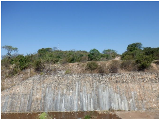
S(3) Spillway Retaining wall (right): Efflorescence from cracks (not draining from drainage holes).
