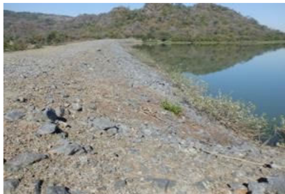
D(1) Embankment Upstream: Disturbance of riprap, dam body exposure and erosion, growth of plants.
