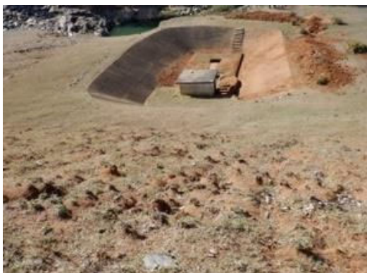
D(5) Embankment Downstream: Eroded soil and sand are flowing to the valve house slope. (Excavating around the valve house.)
