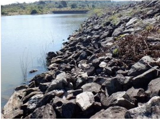
D(1) Embankment Upstream: Exposure of dam body, gully erosion under riprap, and trees.
