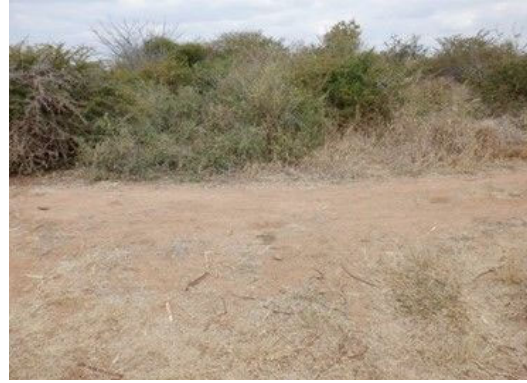
D(8) Left side abutment: Many trees on and around embankment surface (higher than FWL) making it impossible to look out over and pass through. Out side of edge is flat.
