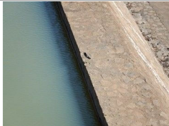
S(2) Spillway weir: Only slight damage (lack of stone) is observed on the top of weir.
