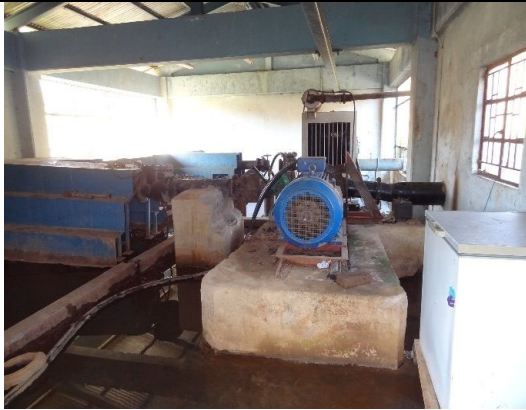
One electric pump equipment has been installed by FAO in 2017.
