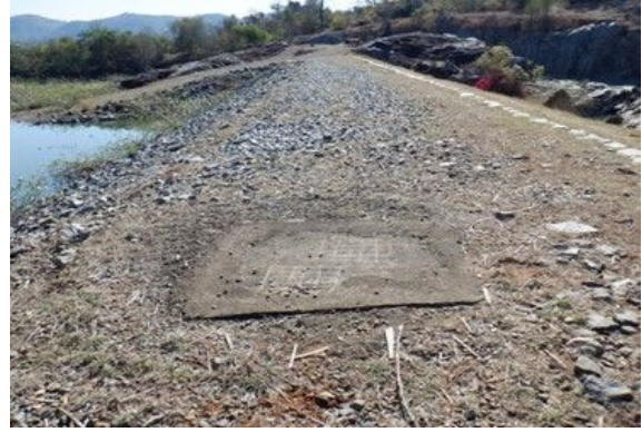
I(1) Intake Inlet: There are no water intake facilities left.
