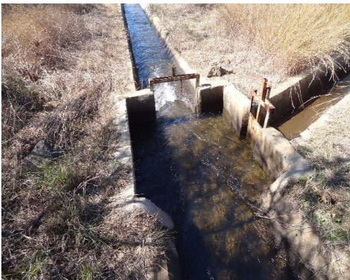
The gate has been lost.
