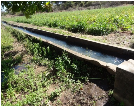
The back soil is flowing out. OF(9):On farm canal(3)
