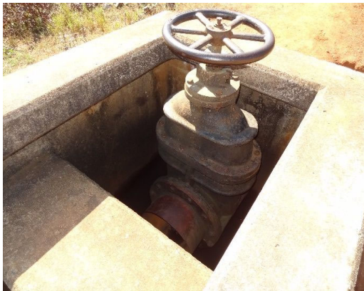
Good condition. OF(3):Night storage(Outlet valve)
