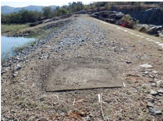
I(1):Inlet: There are no water intake facilities left.
