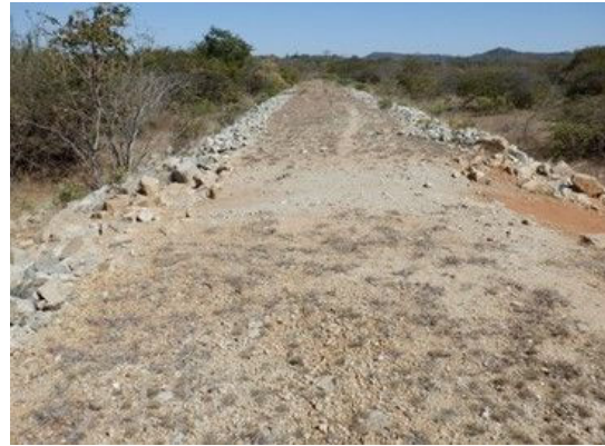
D(8) Left side abutment : No significant damage is observed. The abutment is flat.
