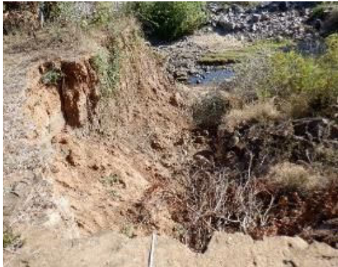
C(5) Connecting Canal: Erosion is also observed on the left bank side (downstream). The bridge has been washed away.
