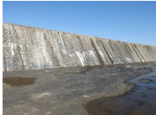
S(2) Spillway 越流堰: There are slight leakages and flows from cracks on the downstream.
