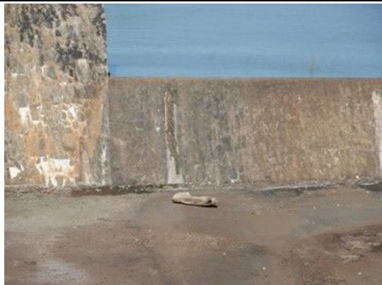
S(3) Spillway weir: There is small leakage from crack on the downstream, no flow can be seen.
