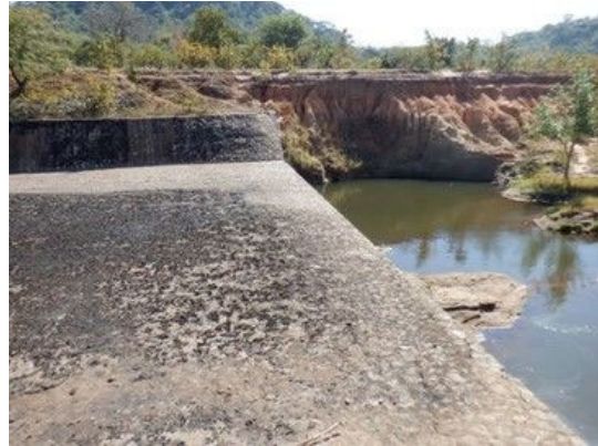
C(2) Connecting Canal(left): Collapses next to the spillway canal, but those does not seem to be in progress(L10.0m,B3.0m,H7.0m).
