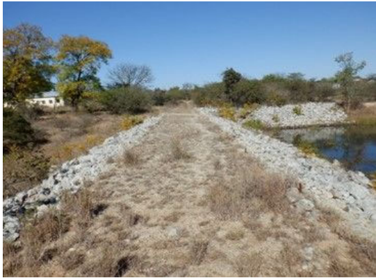
D(7) Right side abutment : No significant damage is observed. The abutment is flat.
