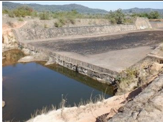
S(9) Spillway canal: There is a slight leak from the back of the canal.
