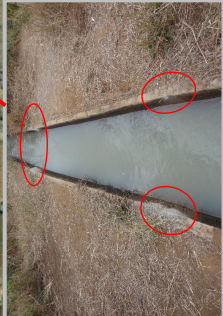
Drainage and Maintained Canal The main canal joint has been maintained by concrete.
