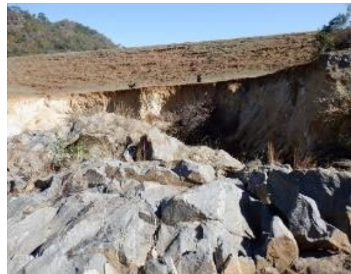
C(2) Connecting Canal: The large erosion is observed on the right bank side (embankment side). According to the existing photo data, the bank is eroded by about 70cm every year.
