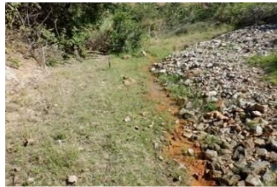
D(10) Foot of slope: In the downstream, a small stream is observed and connects to the connecting canal (on the flowbed, reddish brown and a film is also observed).
