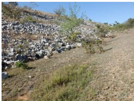
D(4) Embankment Downstream(left): Seepage at the downstream slope edge.
