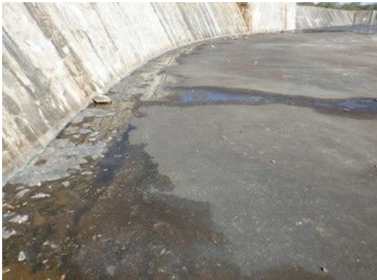
S(7) Spillway canal: There is seepage at joints and the boundary of the retaining wall (no flow is observed).
