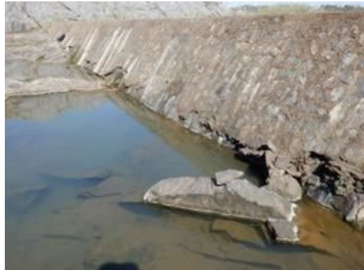
S(4) Spillway Weir: Surface concrete peeling at the downstream of the weir.( h50cm/ t5cm)
