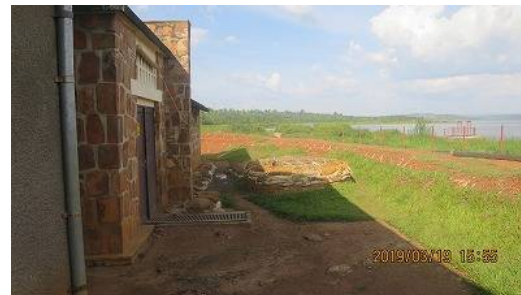
Pump station (left) of Karenge WTP, which is facing the risk of inundation during the rainy season.
