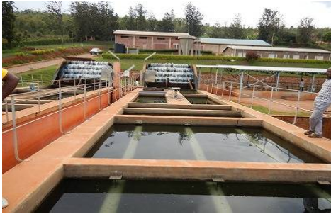
Cascade aeration (in the back), followed by coagulation, flocculation, sedimentation facilities (2 series, 2 basins/series)
