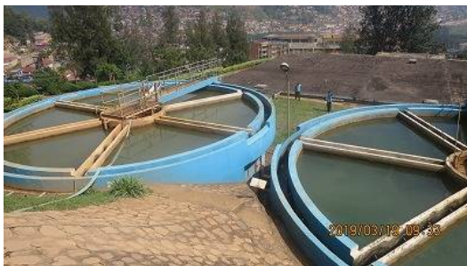
High-rate clarification basins
