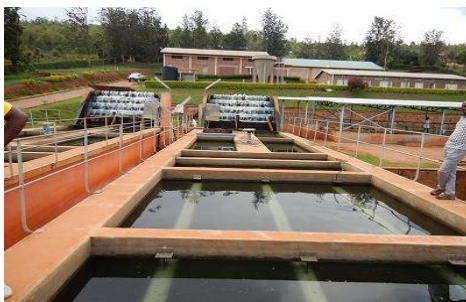
Cascade aeration, coagulation, flocculation, sedimentation facilities (2 series, 2 basins/series) 出典：調査団
