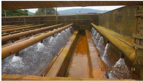
Biological contact oxidation tank
