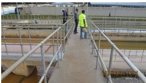
Mixing, flocculation, sedimentation and aeration facilities
