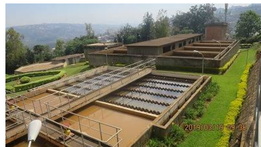
Tube settler sedimentation basins (front) and rapid sand filters (back)
