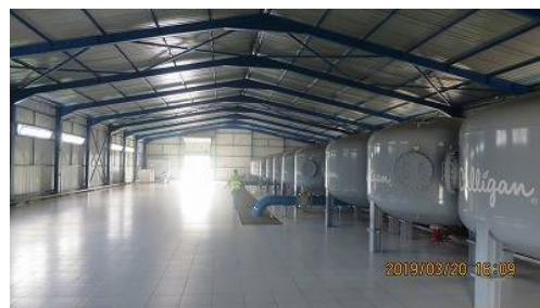
Pressure filters (2 stages filtration, open space on left will be used for installing filters of New Nzove 1 Phase 2
