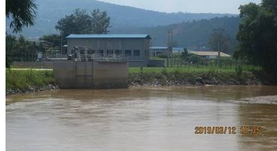
New intake with grit chamber for Nzove 2 WTP (including New Nzove 1 WTP)
