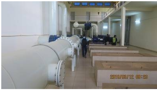
Transmission pump station
