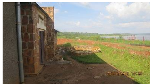
Pump station (left) of Karengye WTP, which is facing the risk of inundation during the rainy season.
