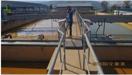
Mixing, flocculation, sedimentation and aeration facilities
