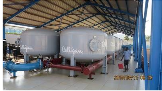
Pressure filters (2 stages filtration)
