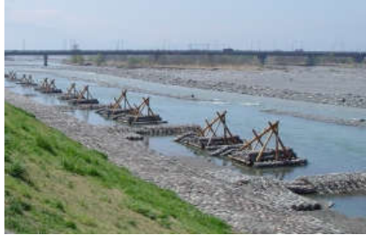
Water Control Work: Sacred Cows (Groyne)
