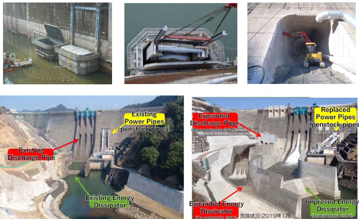
Note: (Upper left and center) upstream coffering, (Upper right) drilling of dam body, (Lower) before and after the works Source: Sendai-gawa River Office, MLIT
