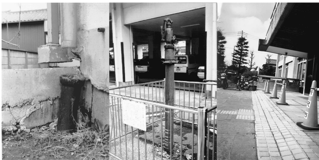
Rising of a Building in Urayasu City, Chiba Prefecture Rising of a Well Pipe in Katsushika Ward, Tokyo Uneven Ground in Tokorozawa City, Saitama Prefecture Source: National Ground Environment Information Directory, Ministry of the Environment
