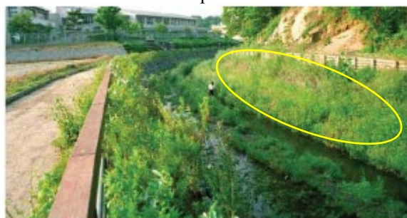
Half year after construction: vegetation recovered on the gabions covered with soils
