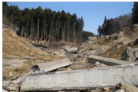
Source: Causes of the Break of Fujinuma Dam, Emergency debriefing one month after the great east Japan Earthquake by Tohoku University
