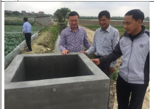
Field instruction and installation of garbage bin for agrochemical package to apply Basic GAP in Quynh Hai cooperative (Thai Binh, 29th January 2019)
