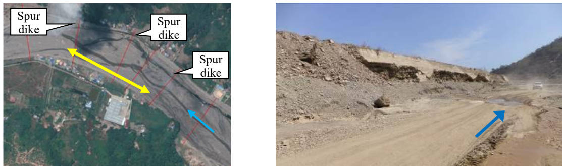
Source: (Left) Compiled by the research team from NTT DATA satellite images, (Right) Taken by the research team Figure 11 Damage to river wall (L3)
