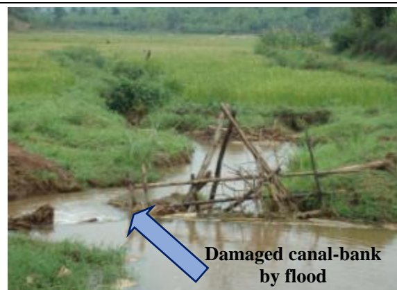
Photo-3 A damaged canal-bank by flood in Gacenshero zone (Mushikiri Rice Growers Cooperative)
