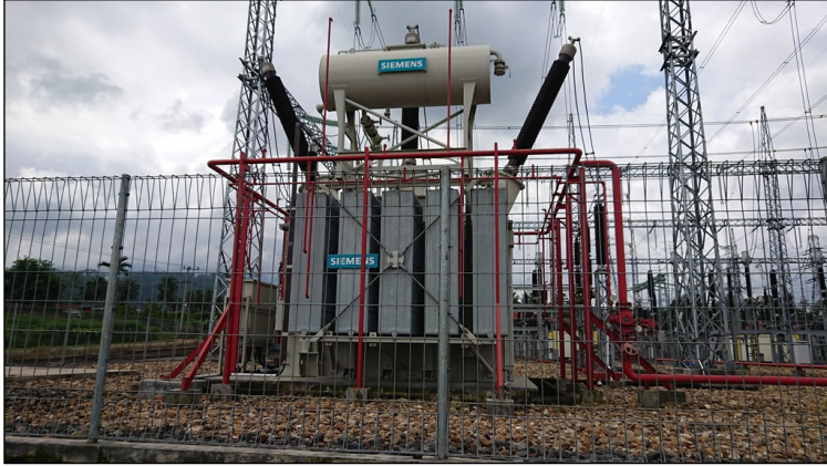
The Payakumbuh Substation expanded by the project (West Sumatra)
