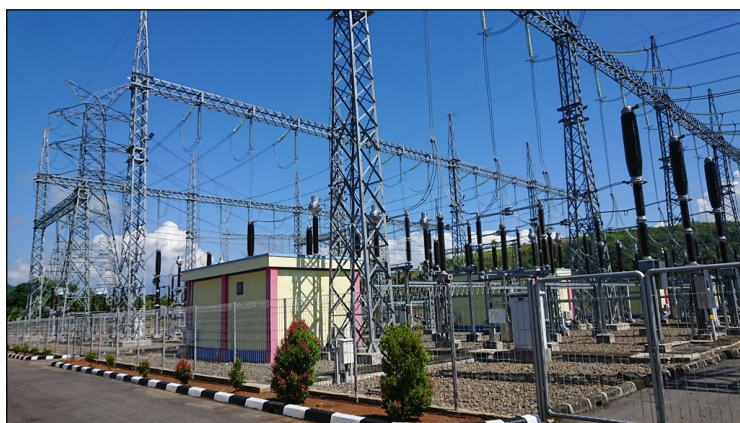
The Padang Sidempuan Substation expanded by the project (North Sumatra)
