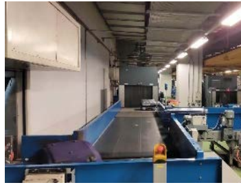
Baggage Handling System
