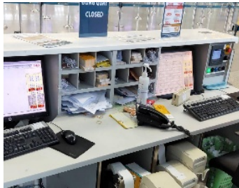
Common Use Terminal Equipment (CUTE)
