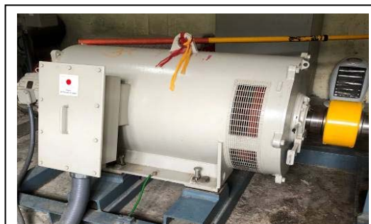
Bajhang Micro-Hydropower Station's Generator
