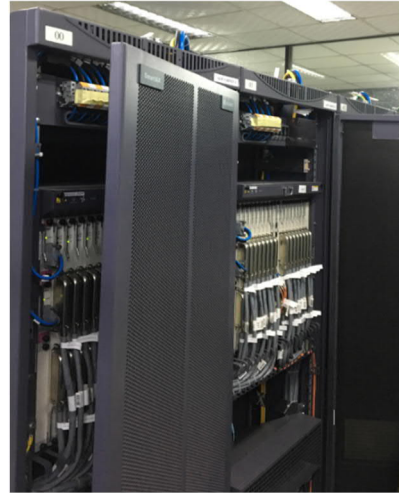
Interface equipment installed in the Project
