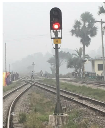
A Signal Installed through the Project
