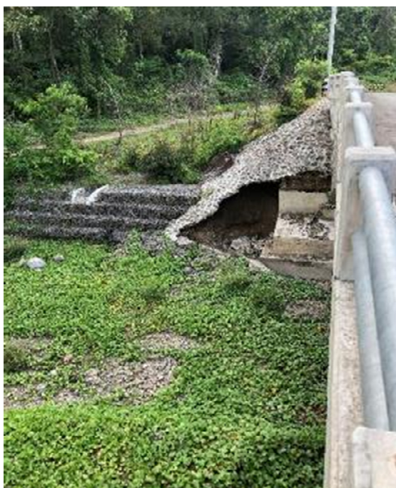
Collapsed Abutment Protection (Mone I)
