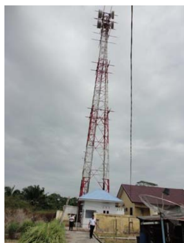
Exterior of Selincing Repeater Station
