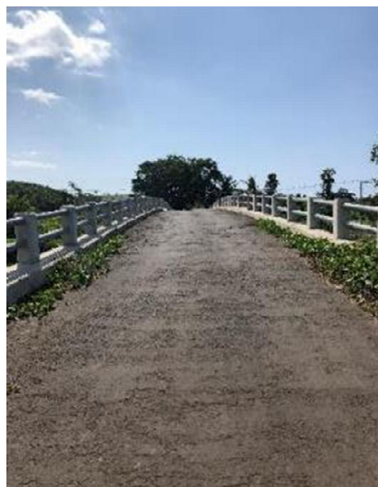
Deteriorated Road Surface (Telonang I)
