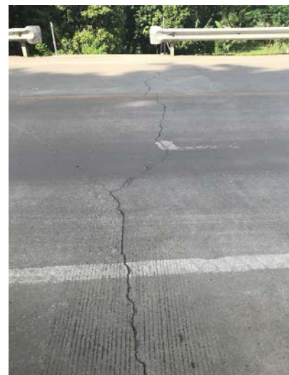
A crack on pavement
