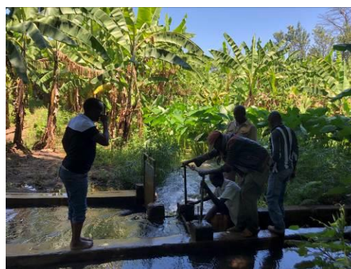
An intake weir constructed by the project and irrigation water users association members
