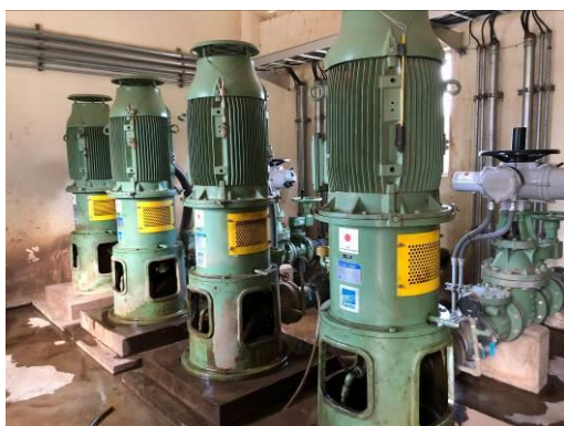
Pumps at the newly constructed intake facilities
