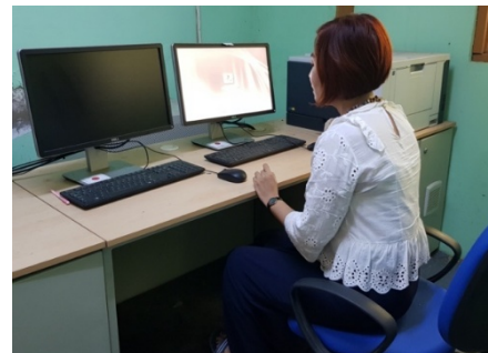
Monitoring equipment for the DMA monitoring system installed in Yegu pumping station
