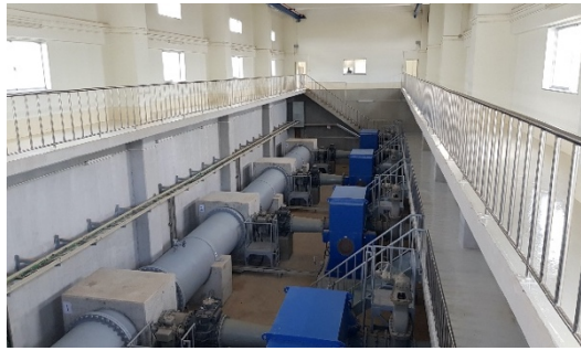
Transmission and distribution pump at the Nyaunghnapin First Phase Water Treatment Plant
