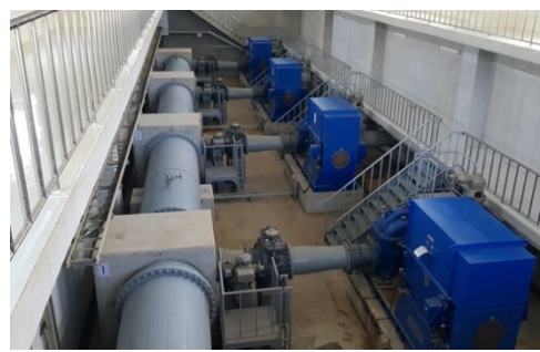
Transmission and Distribution Pump (at the time of ex-post evaluation)
