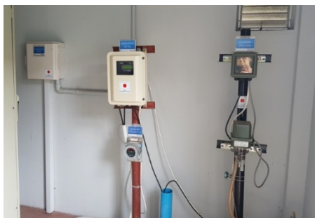
Data recording equipment for DMA monitoring system installed in Yankin Township
