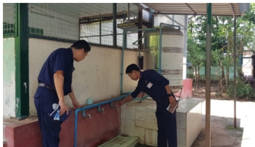
Water pressure and quantity were improved at this primary school in Yankin Township
