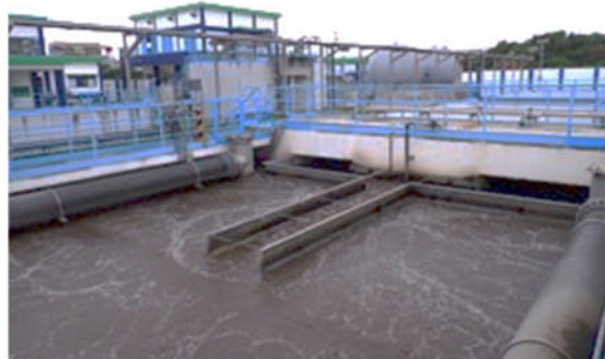
Sewage Treatment Facility Developed by the Project
