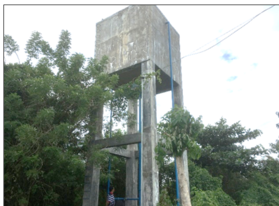
Photo 3: Established Water Supply Facility (Ilocos Norte Province)
