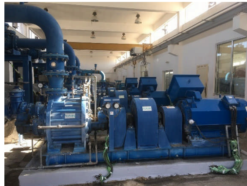
Pumping Station Developed by This Project (Zarqa Pumping Station)
