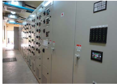
Pump Station Control Room (Battambang)
