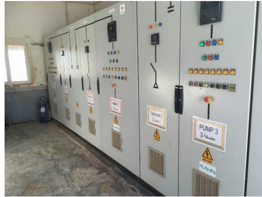
Photo 2: Control System at Azraq Pumping Station
