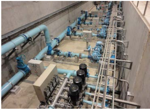
Transmission Pump and Distribution Pump (Battambang)
