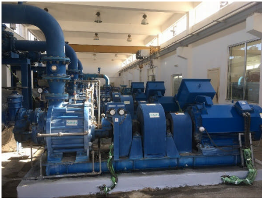
Photo 3: Pumping Facility at Zarqa Pumping Station
