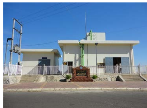
Operation Room of Intake Pump and Generation Room (Exterior of the Building) (Kampong Cham)
