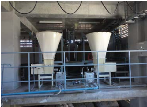
Chemical Feeding Facility (Kampong Cham)
