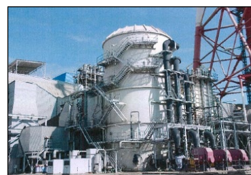
Flue Gas Desulfurization
