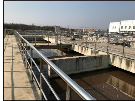
Sewage treatment plant in Nanyang City of Henan Province
