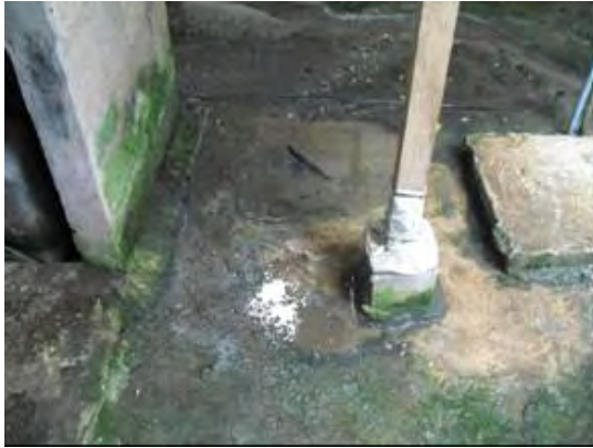
ST and manhole cover for desludging
