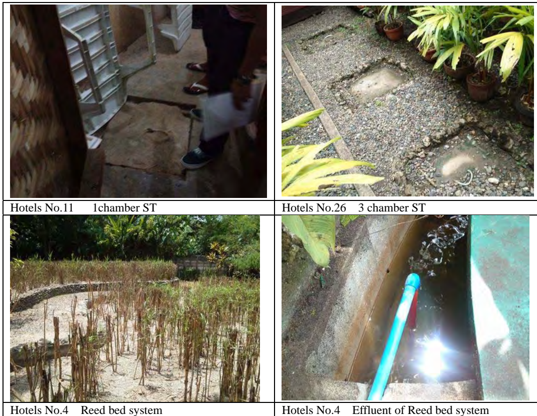
Photo 5.3-4 Individual Treatment Facilities in Dauis (Accommodations)
