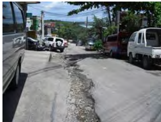
Drains through road surface without drainage system. (intersection of M.H. del Pilar & C. Gallares )
