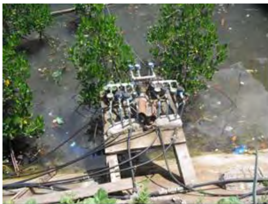
Service connection of water system
