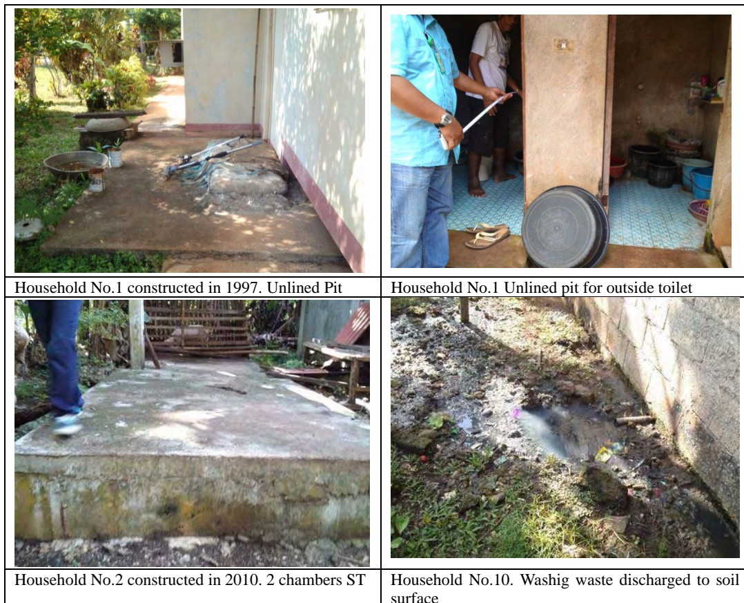
Photo 5.3-3 Individual Treatment Facilities in Panglao (Households)
