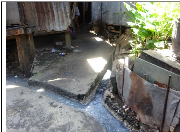
Photo 6.3.2. Narrow and Curving roads where Wastewater flows in Barangay Tomas Monte Verde in Area-A Agdao
