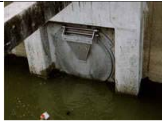
Photo 6.3.5 Example of Flap Gate in a Channel in Japan
