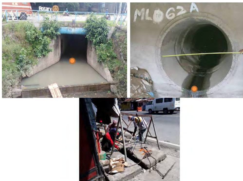
Figure 29: Opening of Manholes in Cainta
