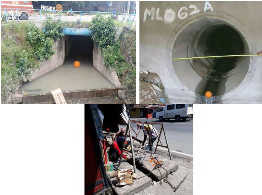
Figure 29: Opening of Manholes in Cainta
