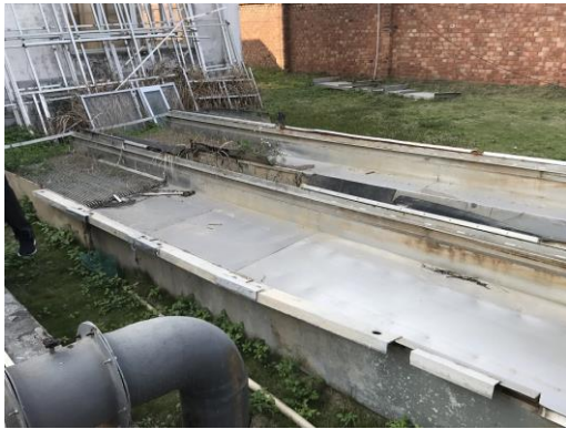
Damaged coarse screen
