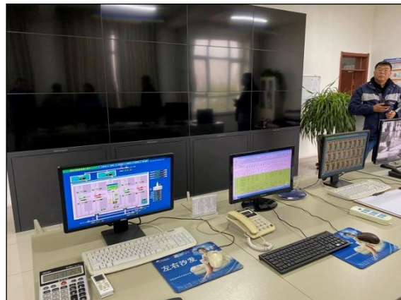
5th Purification Plant (Control Room)
