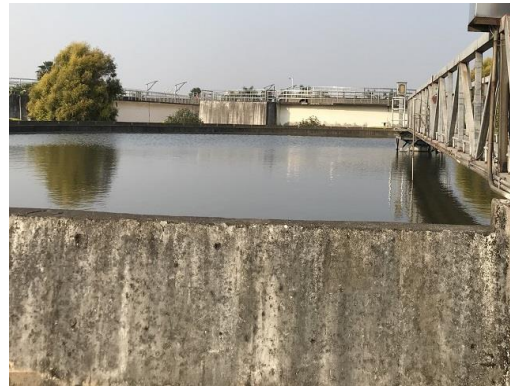
Deteriorated part of concrete structures
