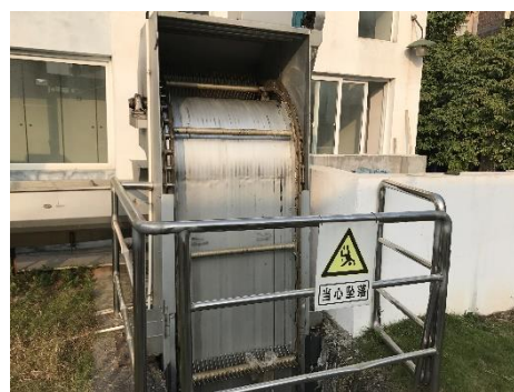
Nanmentang Embankment Sewage Pump Station (coarse screen)
