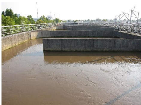
Yulin City Sewage Plant (bioreactor)
