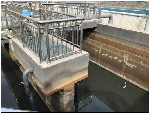
3rd Sewerage Plant Not in Operation
