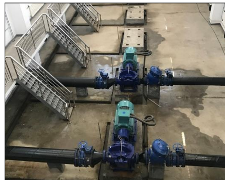
Water Pump System Prepared built under This Project
