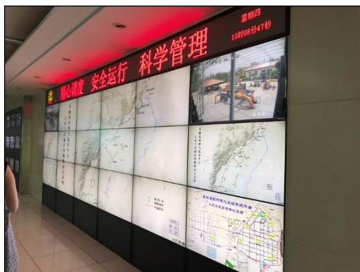
Central Control Room of the Executing Agency (Shizuishan City)
