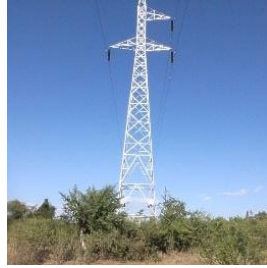
(3) Power transmission lines
