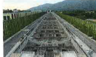
MTR R222/A220 (Dong Kong) Manda constructed an approximately 25 km long section of the high-speed rail that connects between Hong Kong and China's mainland (length approximately 21 km) in length. The section includes a 10 km tunneling section and 5 km cut, in addition, many technologies for site construction including the long side slider system for emergency rescue, rail joints, and electrical cables.
