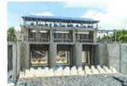
Ayutthaya Flood Prevention Dam (Thailand) Construction of the dam in two sections, from the Canal and the Wang Canal in the East side of the River Chao Phraya in Ayutthaya, courtesy of a grant from the Japanese Government. It includes the construction of an approximately 400 m long embankment on both sides of the river.
