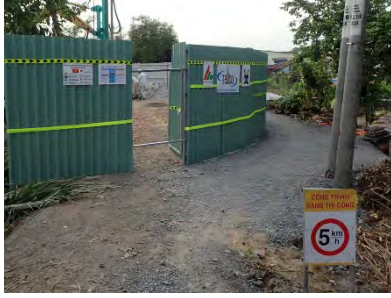
Picture 10. Safety facility (Japanese style)
