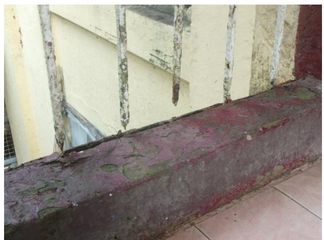
Fracture of baluster in corridor
