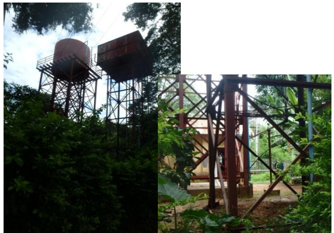
Corrosion of Metal structure of elevated water tank
