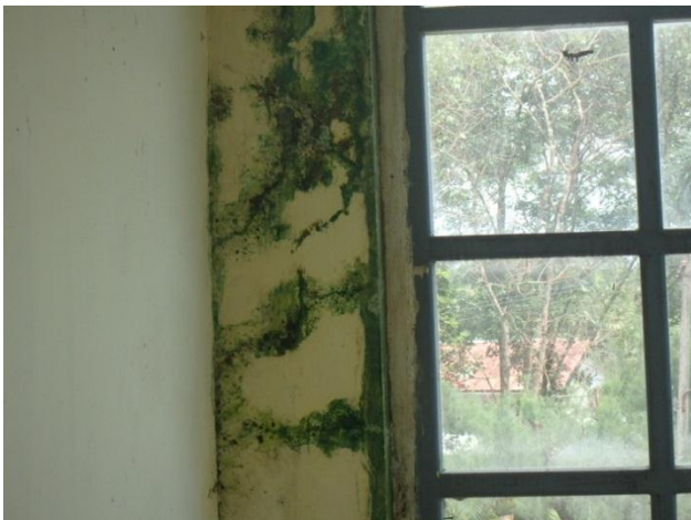
Damage by mold in the staircase in the main building (Constructed in 2003)
