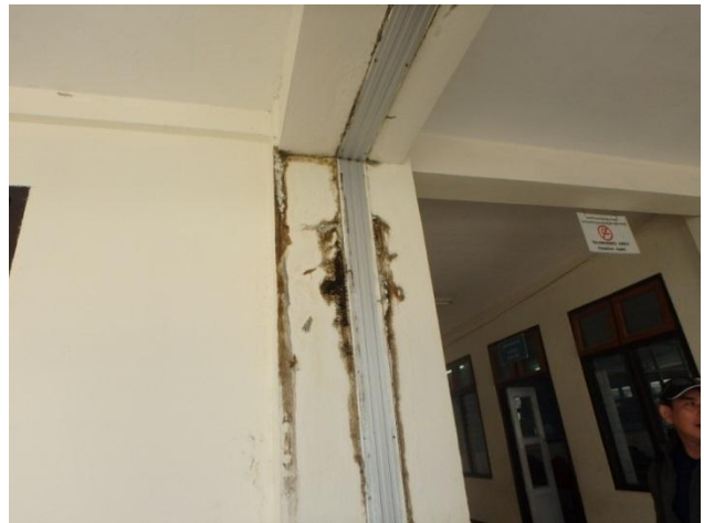
Damage by water leakage and mold at Expansion joint between Building no.4 and 5 (Constructed in 2003)
