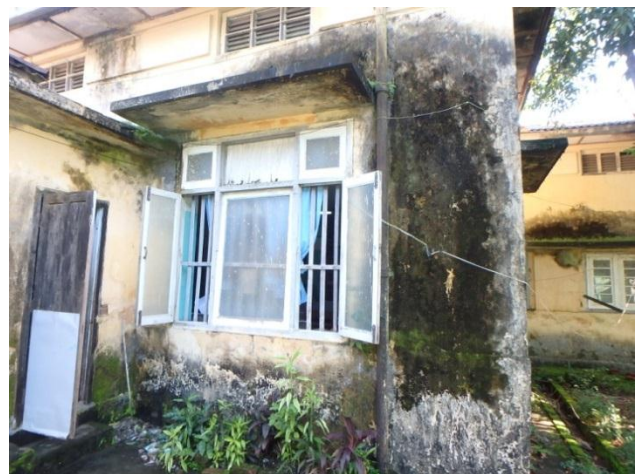
Damage by moss on the exterior wall of building for Administration (Constructed in 1964)
