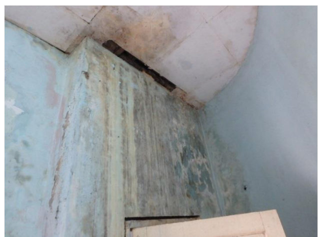
Water leakage at the connection between toilet's roof and sloped roof of Building D
