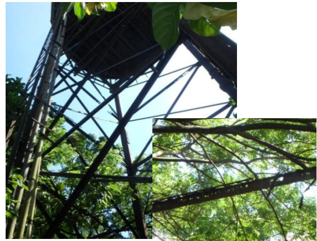
Horizontal steel bars and brace of elevated water tank corroded (Constructed in 1864)
