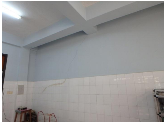
Cracks on the wall of the Delivery room damaged by earthquake (Constructed in 2003)
