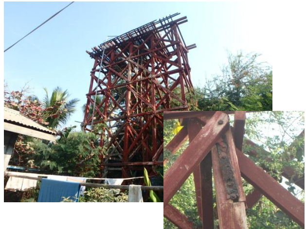
Corrosion of Metal pieces for structural joint of wooden elevated water tank
