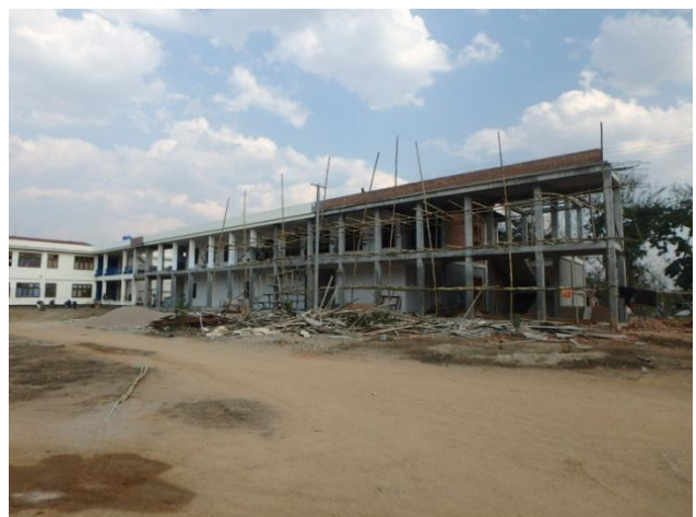
New building under construction for CT scan room, Radiology department and Laboratory
