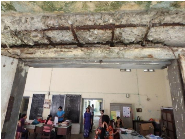
Exposed rebar of lower part of beam at the building for Administration (Constructed in 1964)
