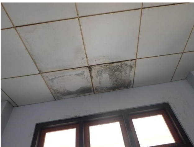
Water leakage on the ceiling at Surgical ward (Constructed in 2003)
