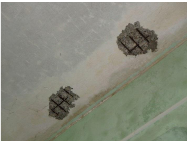
Exfoliation of concrete of floor and exposed rebar at Rehabilitation department (Constructed in 2011)
