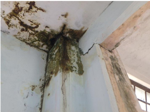
Damage by water leakage and mold at connection between Building no.1 and 5
