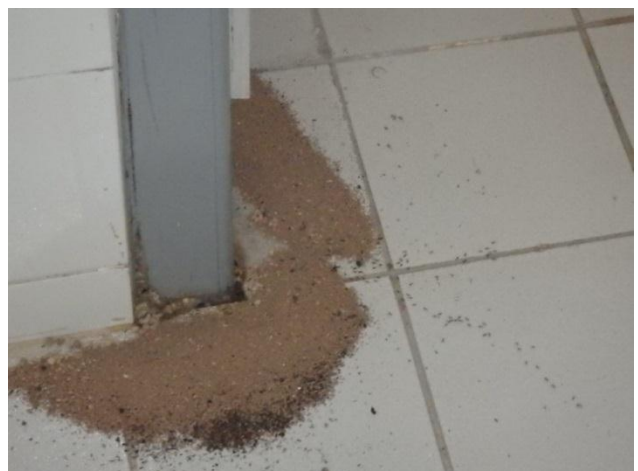
Termite damage in the main building (Constructed in 2003)
