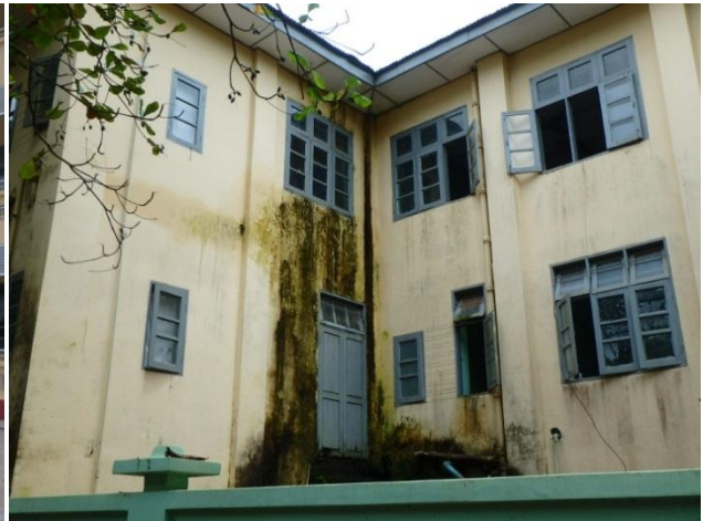
Damage by water leakage and moss on the exterior wall at Ob and Gyn ward
