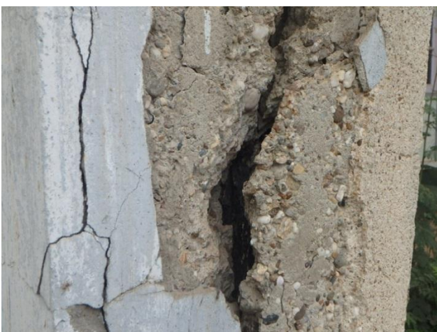
Cracks on the pillar concrete at Building no.7 (Constructed in 1981)
