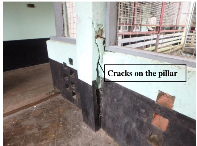
Cracks on the pillar concrete at Surgical ward (Constructed in 1962)
