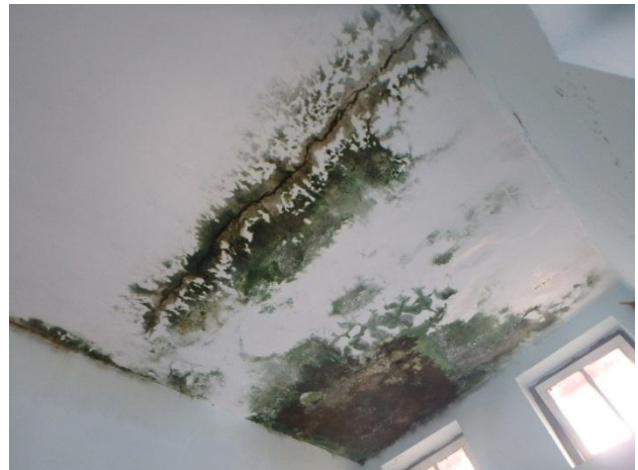
Cracks and mold on the concrete of floor in the toilet at Building no.2 (Constructed in 1990)
