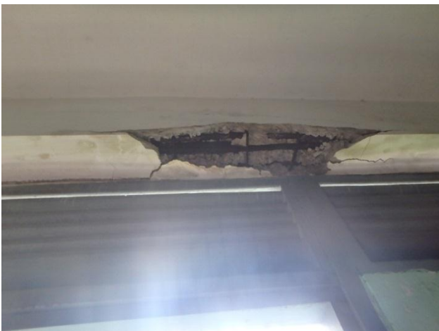
Exposed rebar of the beam in the Orthopedics ward (Constructed in 1962)
