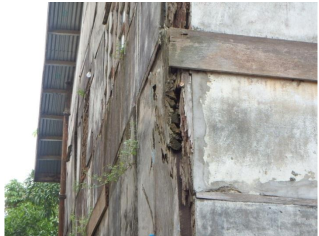
Wooden pillar of old building rotten and risk of collapse at Medical store (Constructed in 1962)
