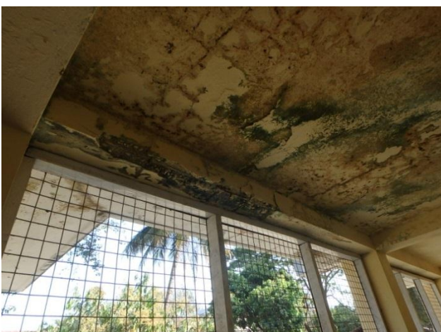
Damage by mold on the slab concrete and exposed rebar in the beam concrete (Constructed in 1966)
