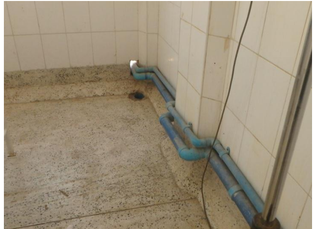
Sewage pipes were installed posteriorly in the Delivery room (Constructed in 2012)
