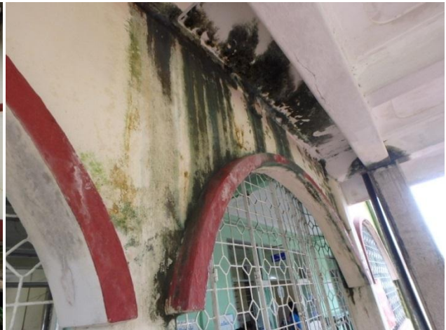
Damage of water leakage, mold and moss on the eaves for entrance of Medical ward
