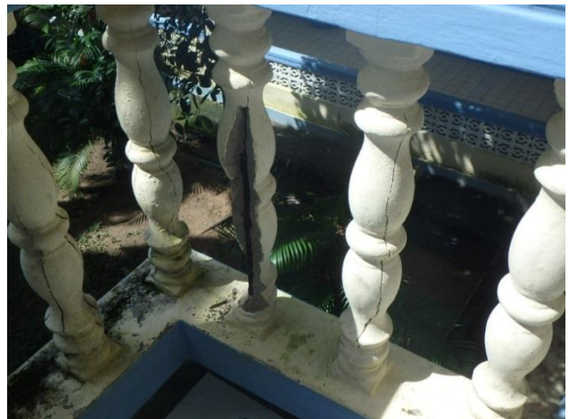
Fracture of baluster in the main building (Constructed in 2003)
