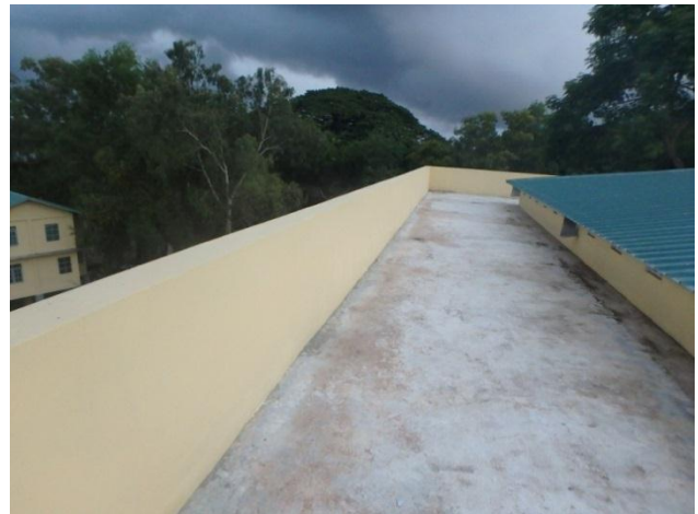
The rooftop of the newest building is not waterproofed (The building for Pediatrics ward constructed in 2014)
