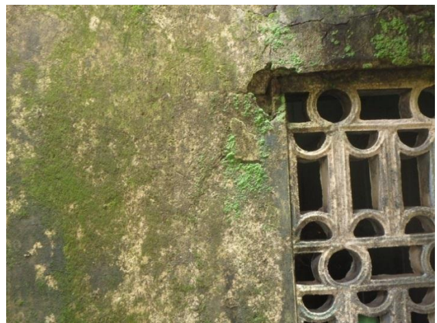
Degradation of exterior wall at Medical ward (Constructed in 1962)
