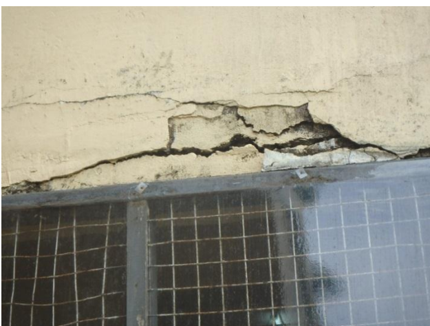
Damage by cracks of concrete on the exterior wall
