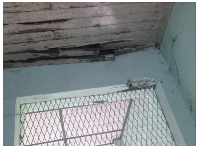
Degradation of ceiling and fracture of concrete
