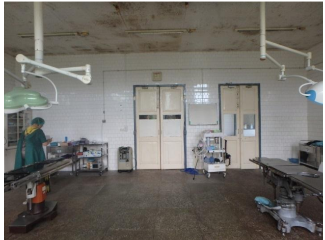
Damage by mold on the ceiling in operation theatre
