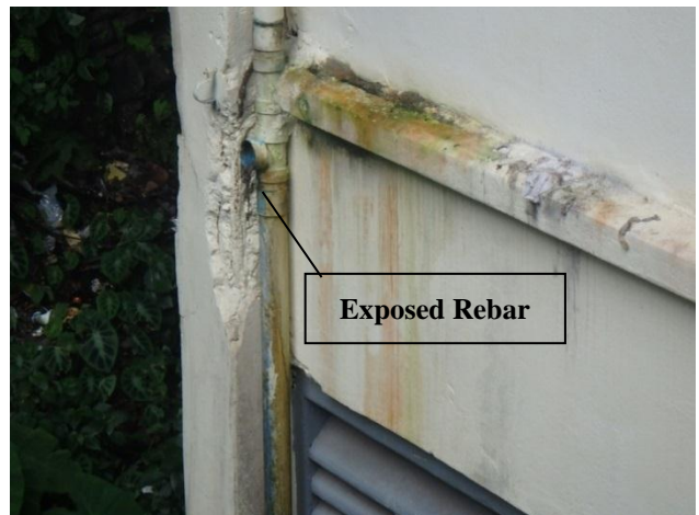
Exposed rebar and a lack of hoop reinforcement at X-ray department (Constructed in 1962)
