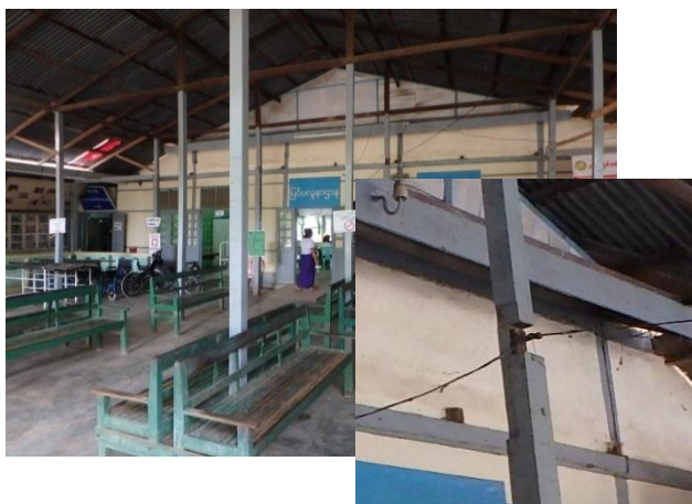
Fracture of wooden pillar at reception and waiting area for Outpatient department
