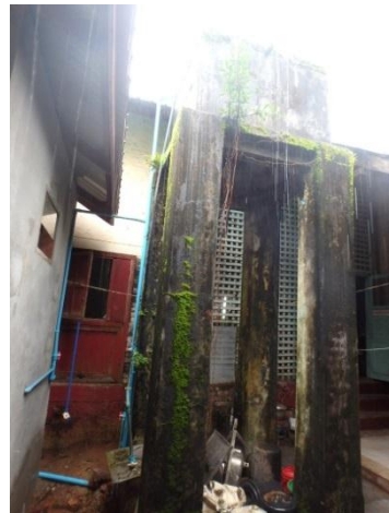
Elevated water tank has been located next to the Laboratory and still used.
