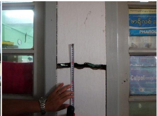
Fracture in the pillar with 30mm's width by uneven settlement at Surgical ward (Constructed in 1973)
