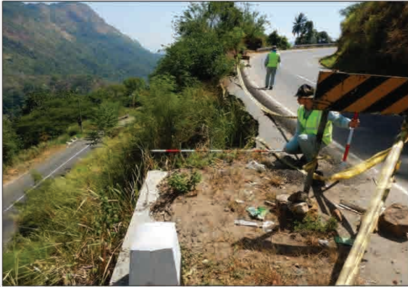
P1 The slope failure occurring along the shoulder on the valley side slope of the road
