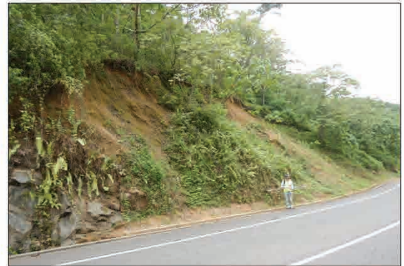
P3 The slope failure occurring on the cut slope above the road (failure high: about 15m)
