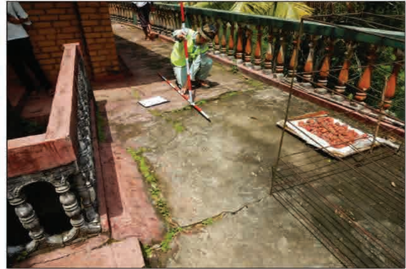
P3 Cracks observed on the house guard above the landslide area
