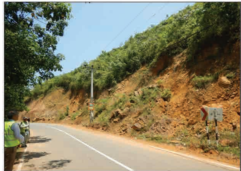
P4 Local surface failures occurring on the cut slope above the road.
