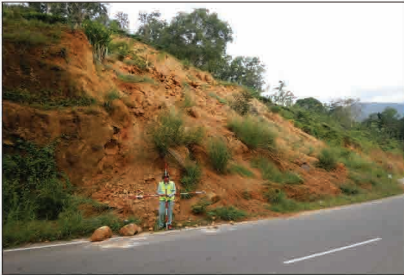
P1 Whole view of the slope failure looking upper slope from the road
