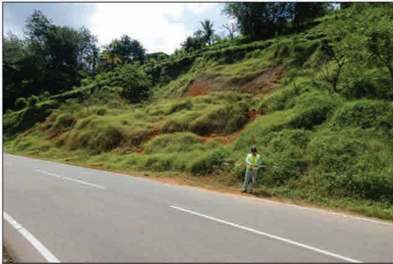
P1 Whole view of the landslide occurring on the cut slope above the road
