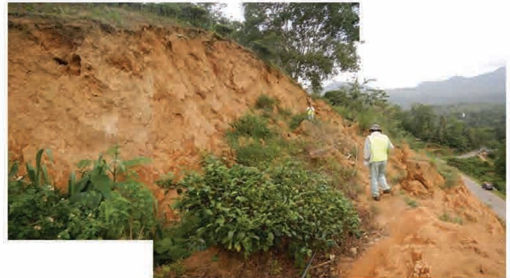
P3 The main scarp of the slope failure (scarp high: about 6m)
