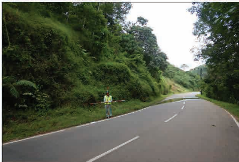
P2 The deformation situation of the cut slope above the road, showing abundant springs
