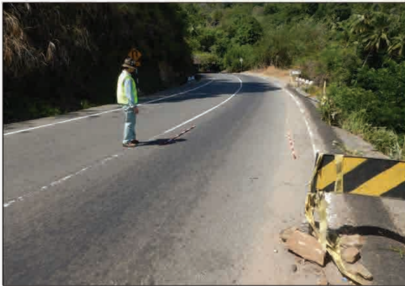
P2 Cracks observed near the central line of the road, showing a potential for further slope failure
