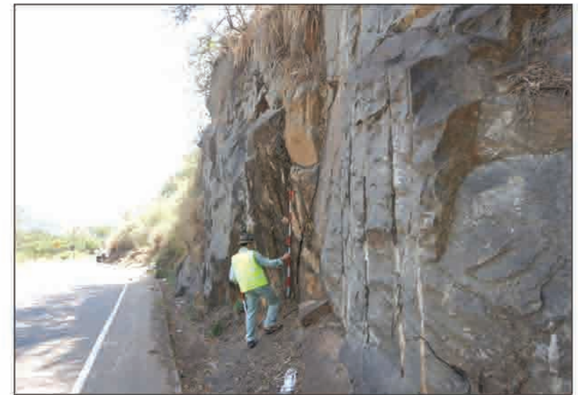
P4 Near-vertical joints observed near the slope failure, showing potential vertical failure surface
