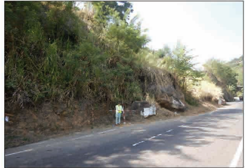
P3 The collapsed materials reaching the central line of the road
