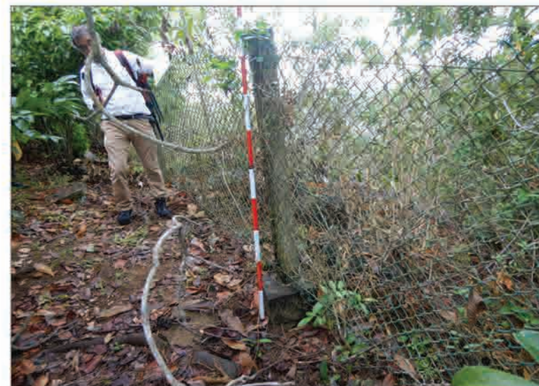
P4 Unstable stones (at max size, \phi 20 \times 50 \times 80 cm), distributed around the ROW boundary fences of RDA.
