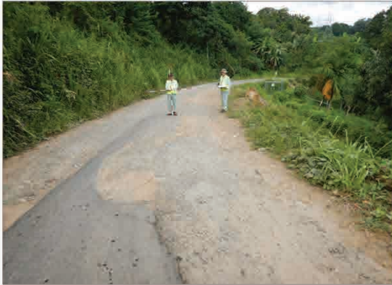
P1 The deformed situation of the village road on the upper slope of the landslide
