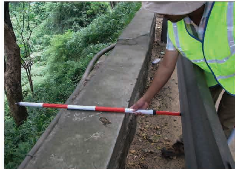
P2 Deformed concrete wall due presumably to movement on the valley side of the road.
