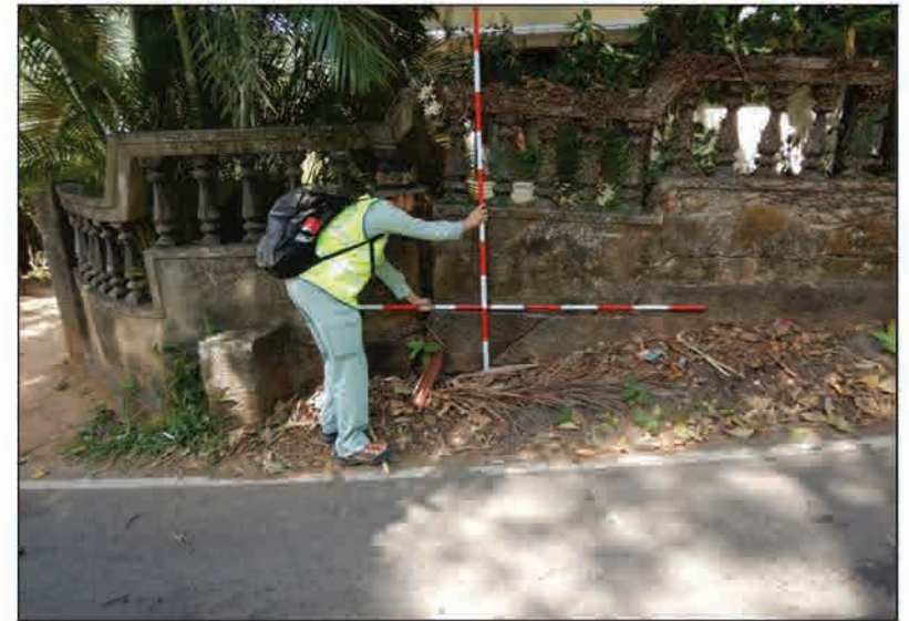
P3 Cracks occurring on the retaining wall within the landslide
