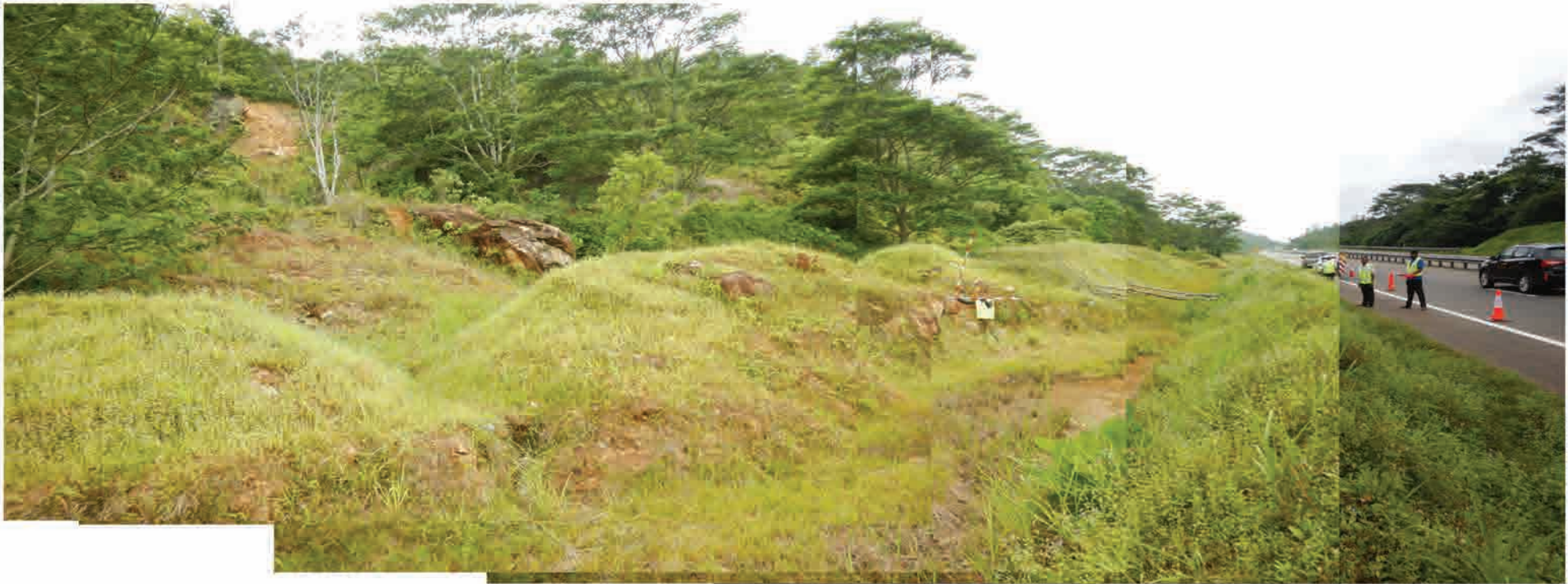
P5 Whole view of the slope failure looking upslope from the road
