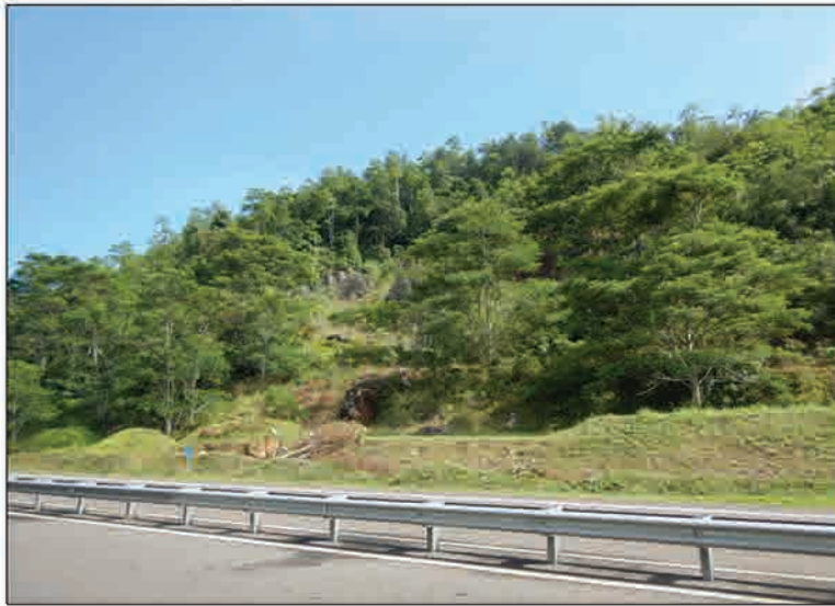
P1 Whole view of the slope failure, the collapsed materials were partially removed and partially flattened on the toe of cut slopes
