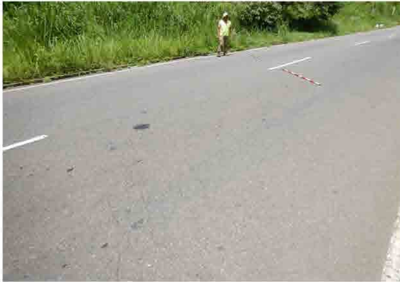
P1 Cracks across the road due presumably to landslide movement
