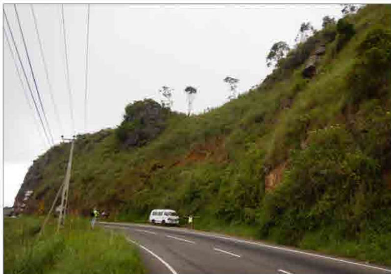
P1 Shallow failure on the cut slope above the road and some individual huge rock blocks on its upper natural slope
