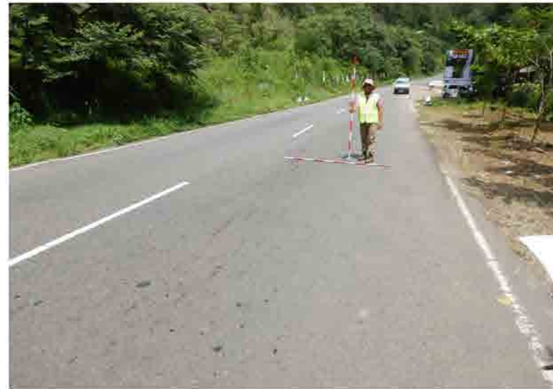
P2 Cracks across the road
