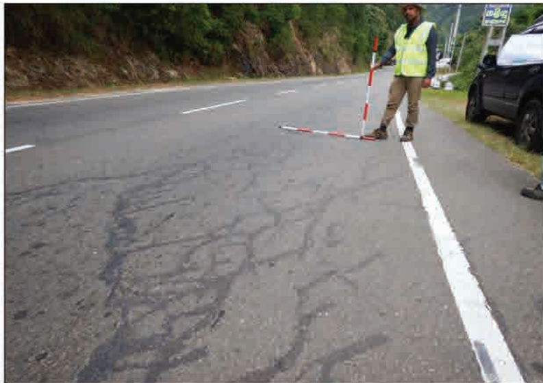
P2 Cracks and deformation situation of the road surface
