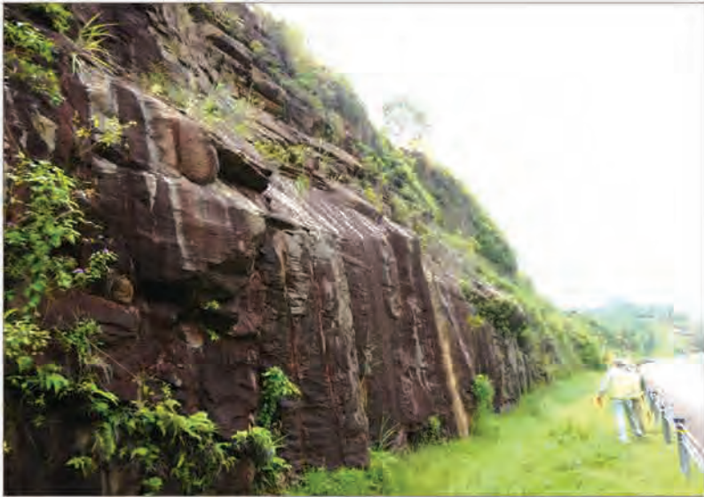
P5 Fractured rock slope, showing a dip slope - high potential for further rockfalls
