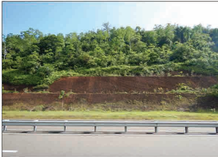
P2 Road cut slope of the strongly weathered rocks next to the slope failure
