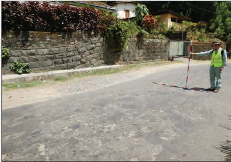
P1 The subsidence of the road surface and the deformation of masonry retaining wall within the landslide
