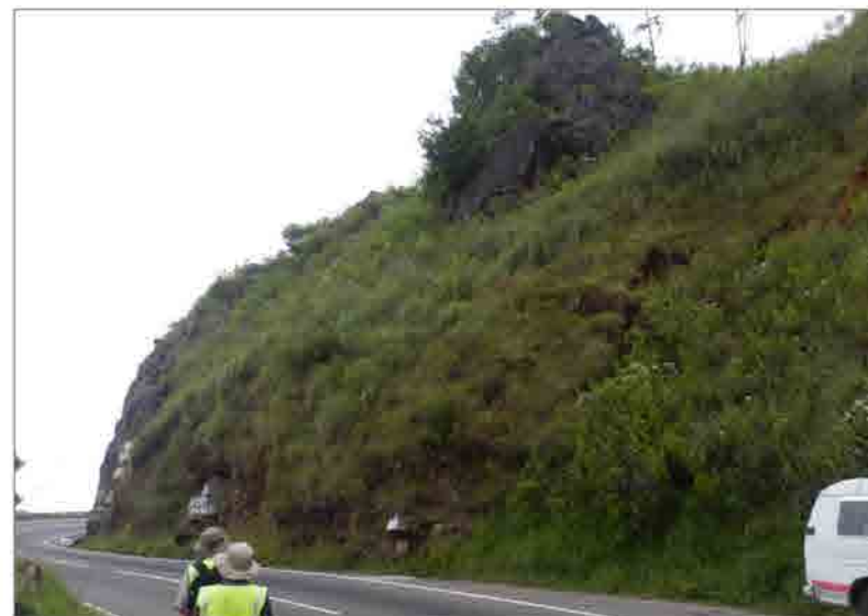
P2 Close view of P1, showing that shallow failure would contribute to potential for falling of huge rock block on its upper natural slope
