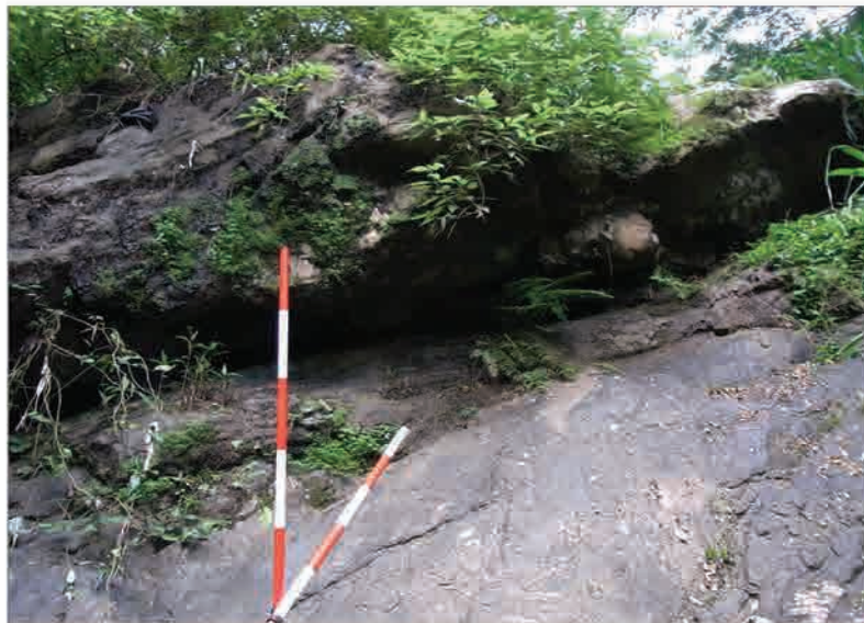
P3 Open cracks observed below the road
