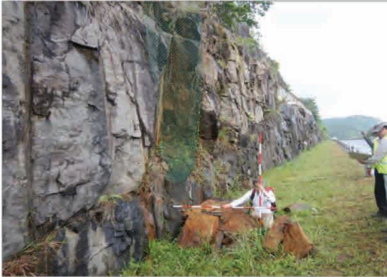
P1 Huge rock blocks falling due to wedge rock failure on the rock cut slope
