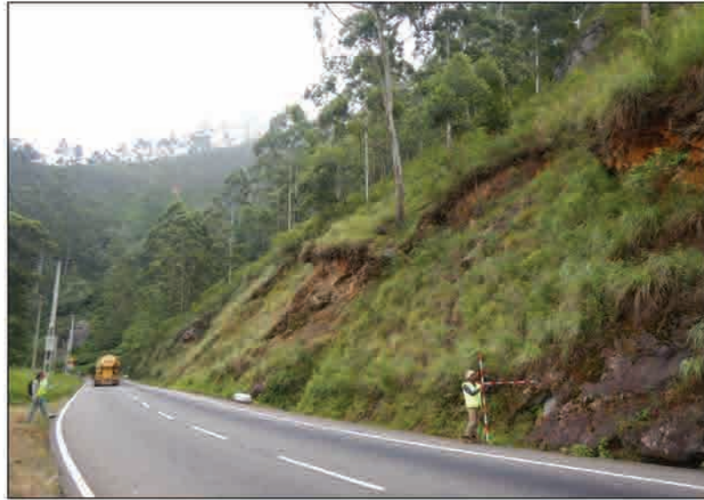
P5: The surface failure of cut slope
