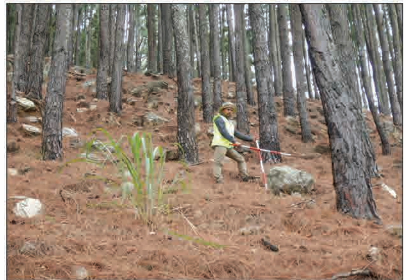
P4 Numerous boulders distributed on the upper slope of the road cut slope (diameter 60cm )
