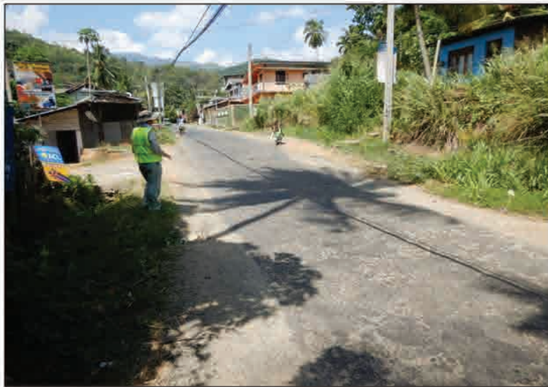
P2 The deformation situation of the road that pass along the middle part of landslide
