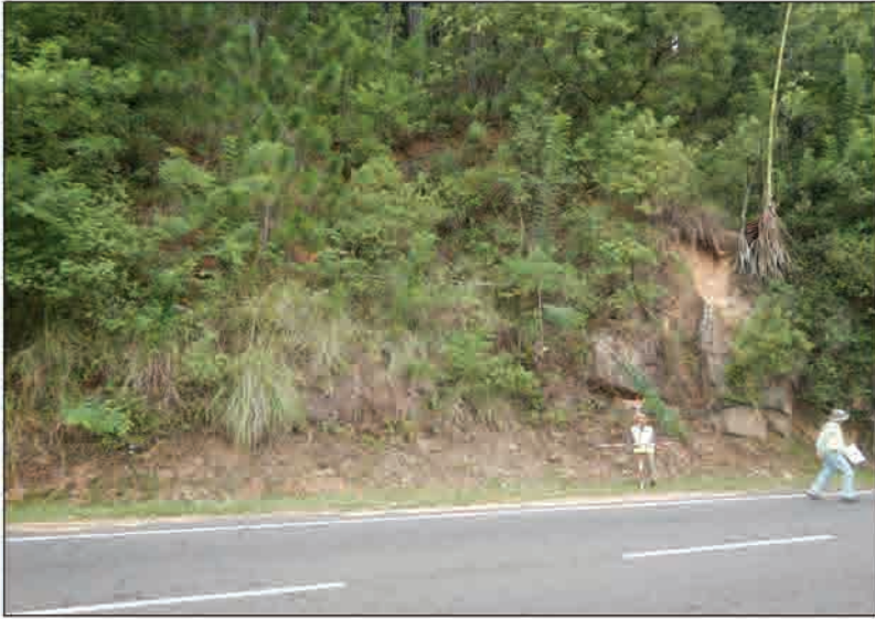
P1 The cut slope situation of the target section
