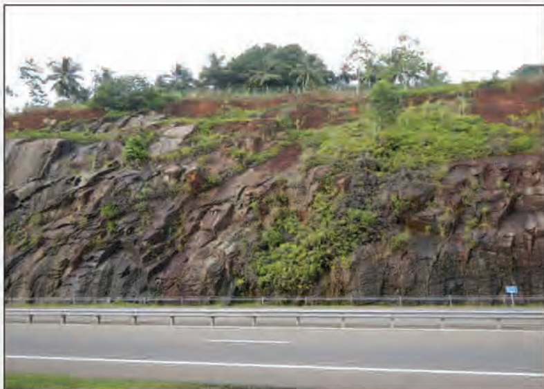
P5 Similar to that in P4, showing major joints dipping out of the cut slope in the slightly weathered rocks, further indicating a high potential for rockfalls
