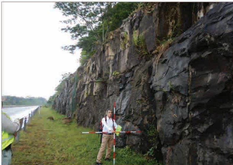
P2 Major joints dipping adversely out of the cut slope, showing high potential for rockfall
