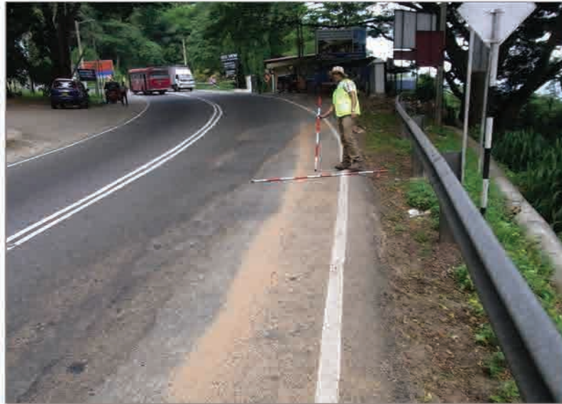
P1 Deformation situation of the road surface on the valley side of the road
