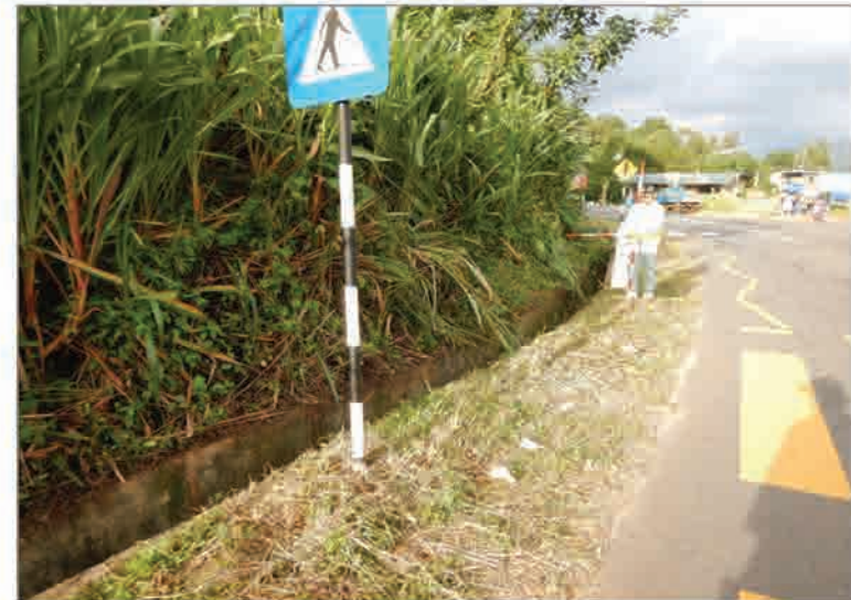
P4 The landslide toe along the road side ditch
