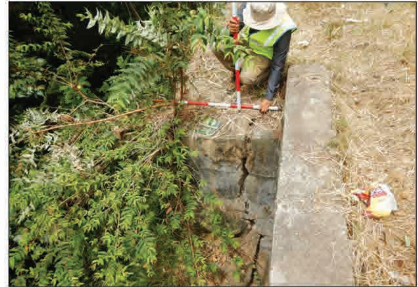
P3 Cracks occurring on the block wall on the valley side of the road
