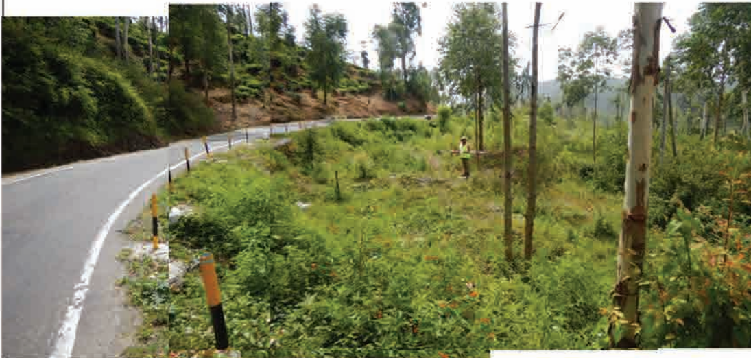
P3 Circular depression just along and below the road due to landslide movement
