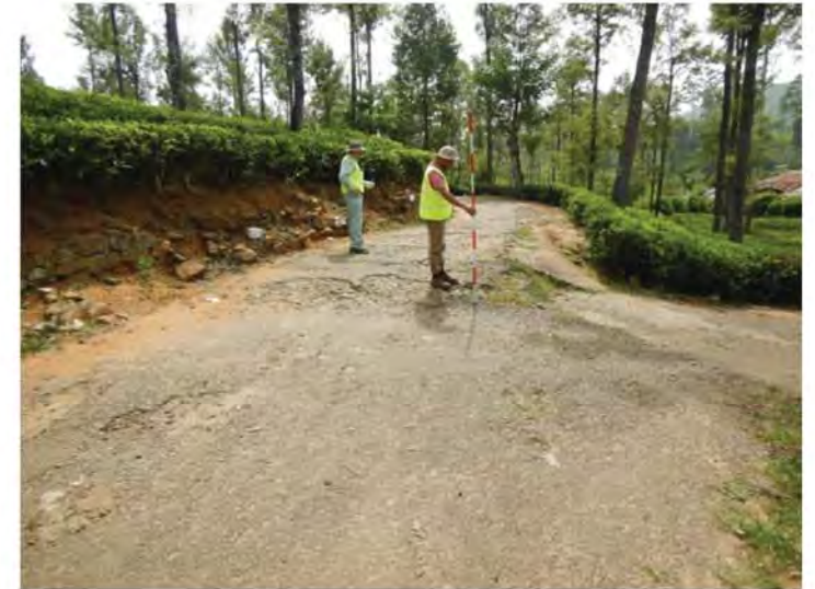
P6 Deformation and upheaval situation of the village road around the the toe of landslide
