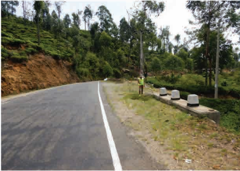
P1 The upper slope of the landslide area looking from the starting point of the road.
