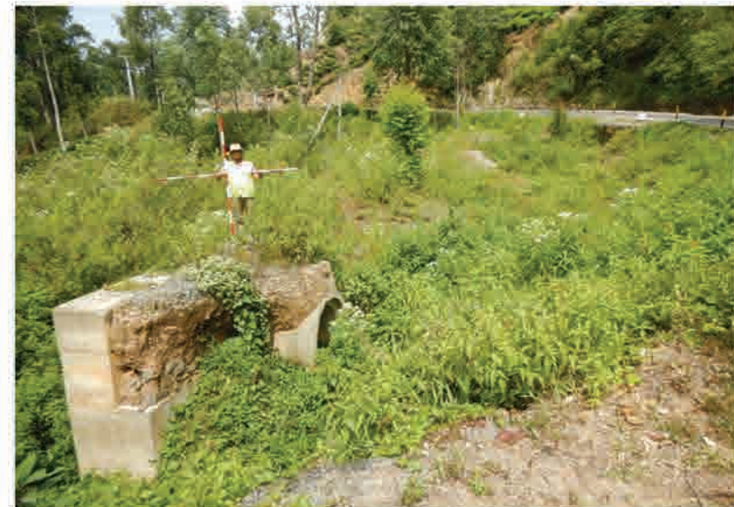
P4 Culvert destroyed by landslide movement
