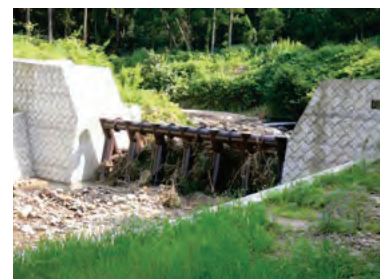
Permeable Sabo dam
